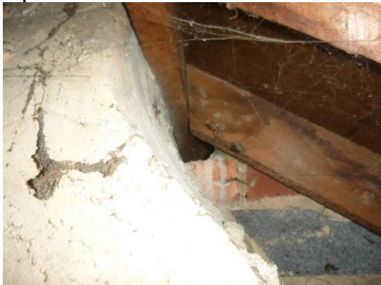
17. Gap into neighbouring void next to chimney.
