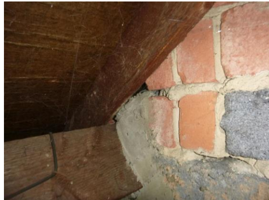
18. Gap behind end rafter at party wall.
