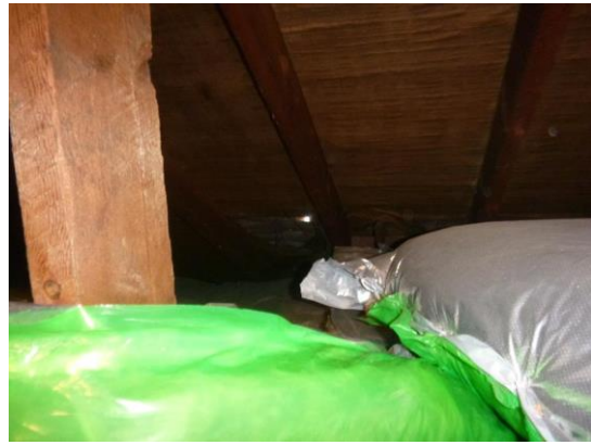
14. Daylight visible at front bay window.
