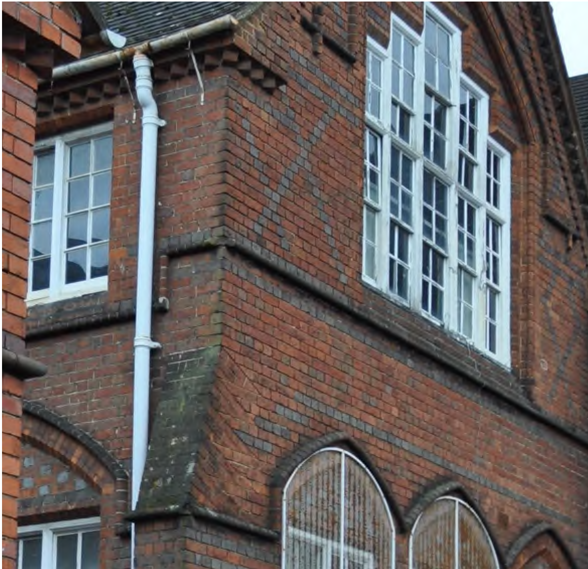
1.4.4 Brickwork W1 Gable – broken string course corner bricks and differential joint weathering
