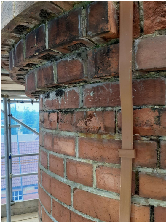
Figure 9. Detail of segregating ring between upper parts 2 and 3. Local vertical cracks on upper part 2.
