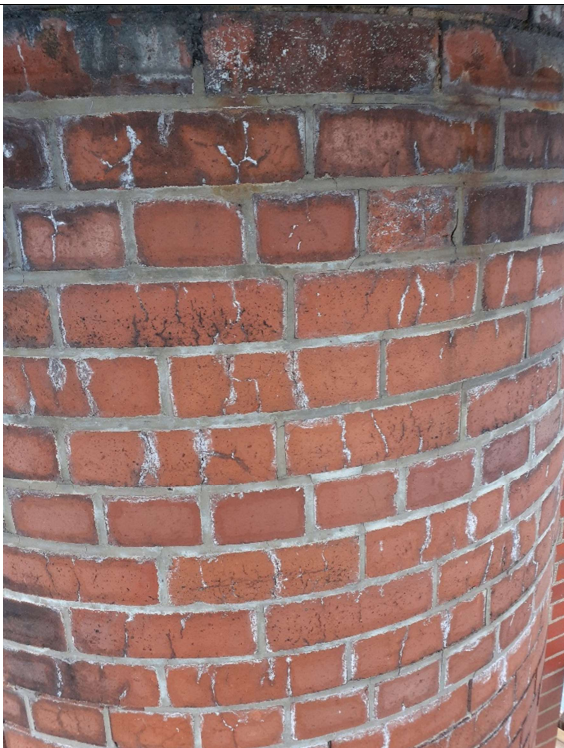
Figure 12. Upper English bond build-up parts.
