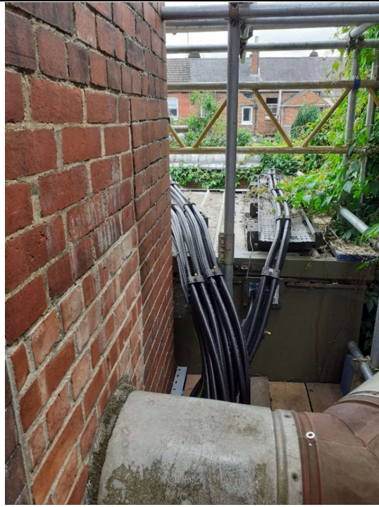
Figure 6. View from first scaffold level. Remaining ventilation pipe (front), cabinet and cable feeders (back)
