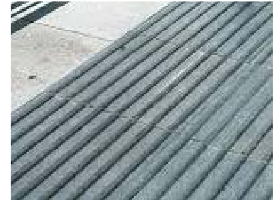
Hazard paving to top and bottom of steps.
