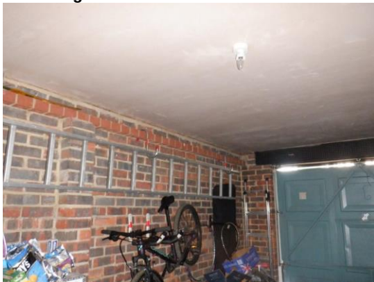
23. Plastered ceiling of garage tight to brickwork.
