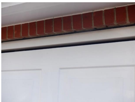
9. Gap above garage doors (front elevation).
