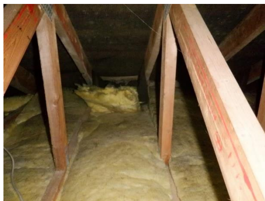
14. Loose bitumen roofing felt around chimney at northern hipped end.
