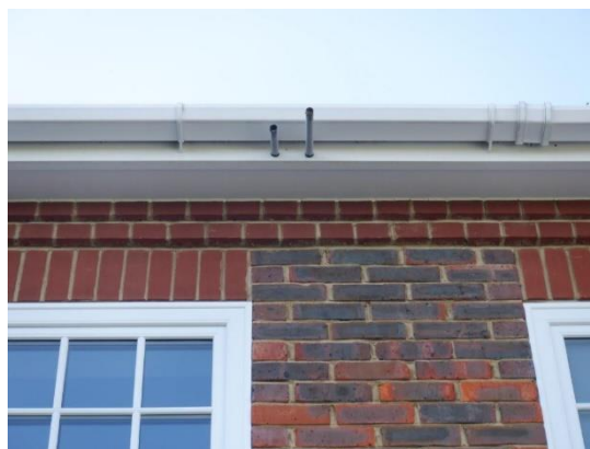
8. Overflow pipes out of uPVC soffit (rear elevation).
