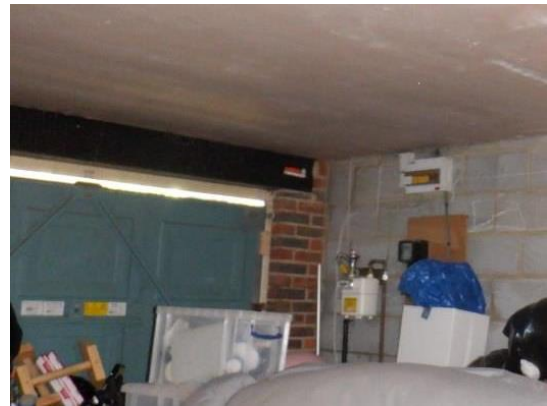
24. Daylight visible above garage doors, which were cobwebbed.
