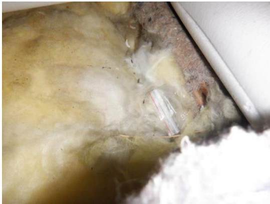
21. Occasional mouse droppings on fibreglass insulation.
