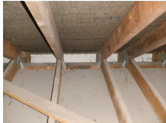
22. Open eaves into soffit.
