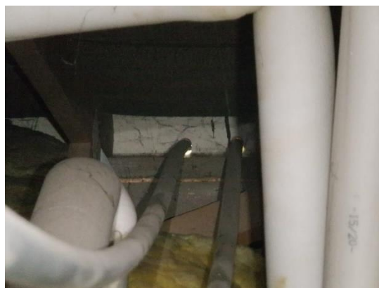
16. Daylight visible around overflow pipes in soffit on rear elevation.
