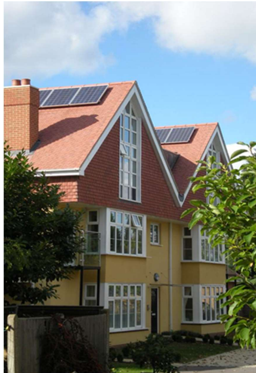
Figure 4: Solar PV installation on an apartment development in Oxford
