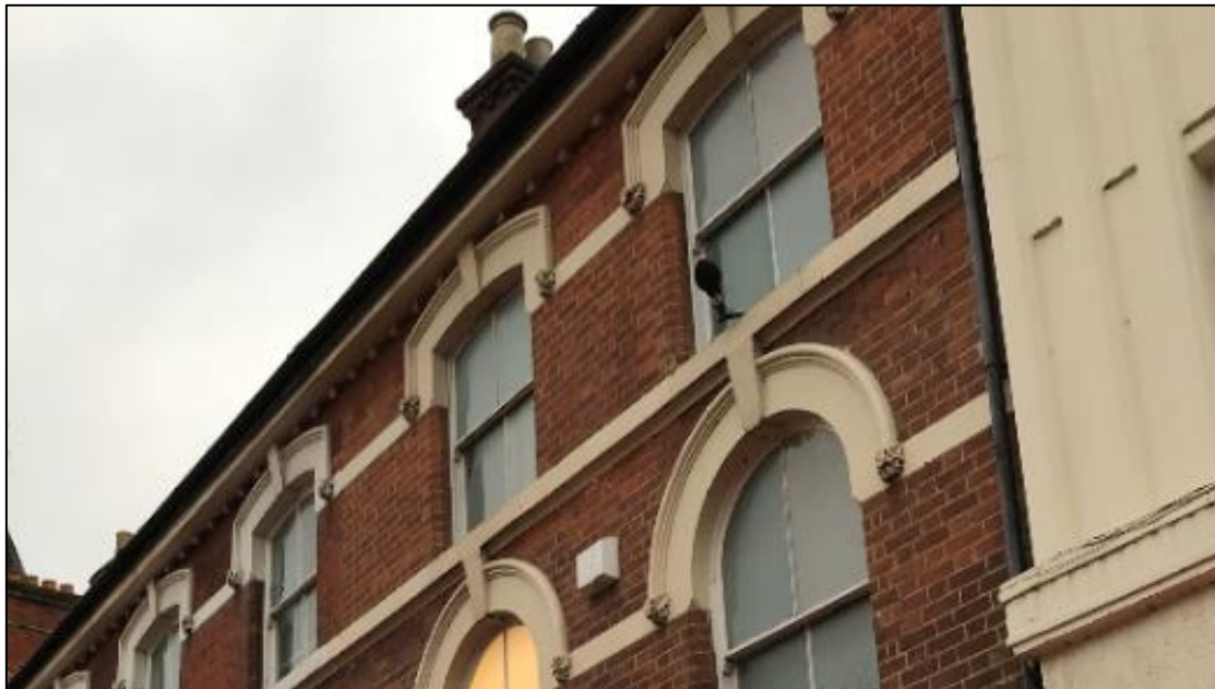
Figure 3 Logger installed on site at position A
