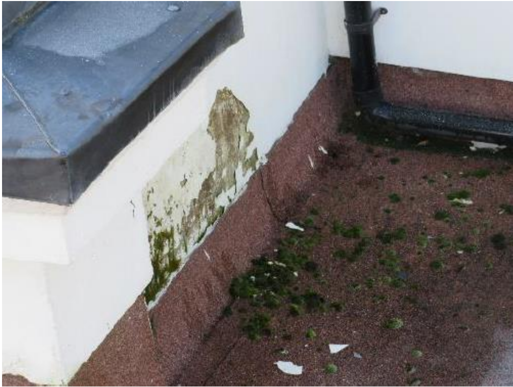
Photo 4 - Disrepair to paintwork/render above lower flat roof to right hand side
