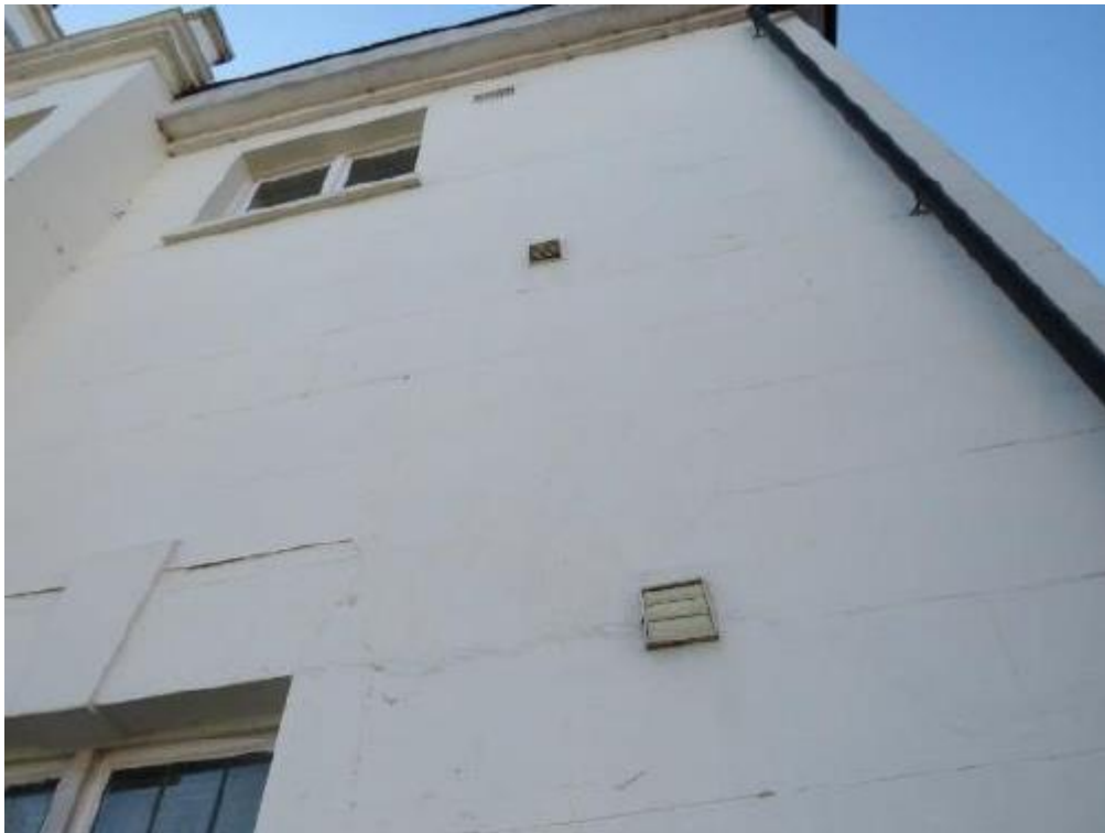
Photo 7 – Hairline cracking to render to right hand elevation
