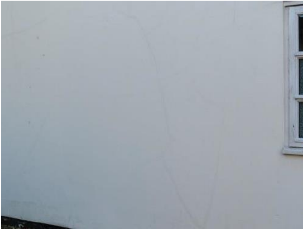
Photo 6 – Typical hairline cracking to render
