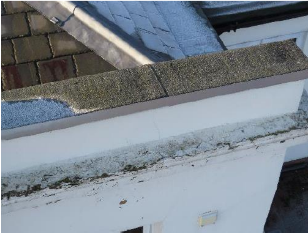
Photo 2 – Right Hand Parapet to Main Roof. Breaking up of render to cornice
