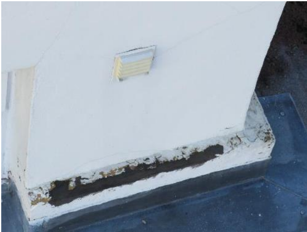
Photo 3 – Typical poor cement render repair and hairline cracking to stucco
