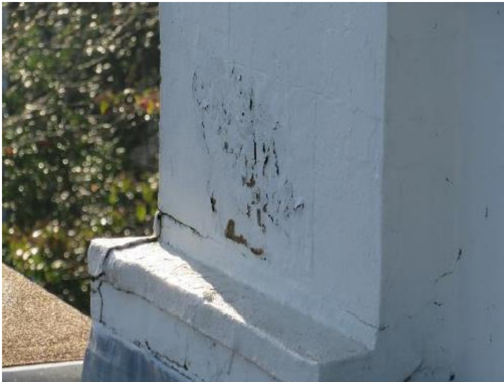
Photo 5 – Typical disrepair to stucco render
