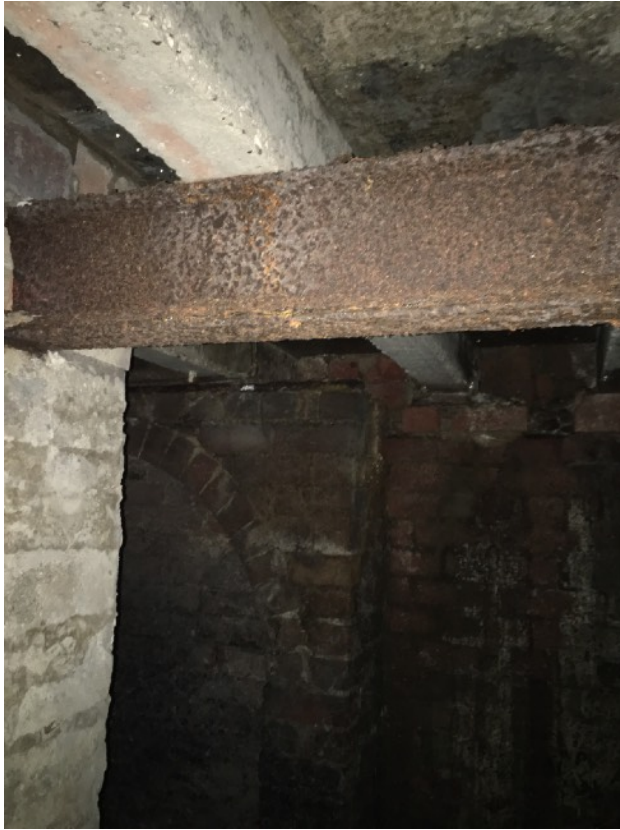
Photograph showing existing steel structure which is in a poor condition and is intended to be replaced
