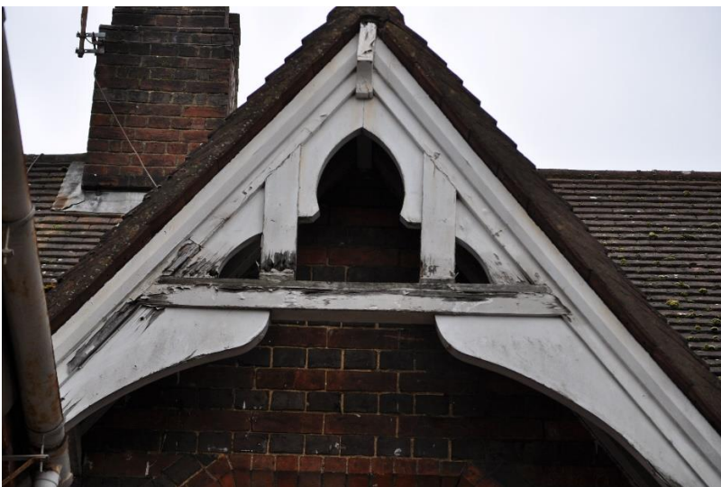
Fig 13 West facing gable woodwork suffering from decay.
