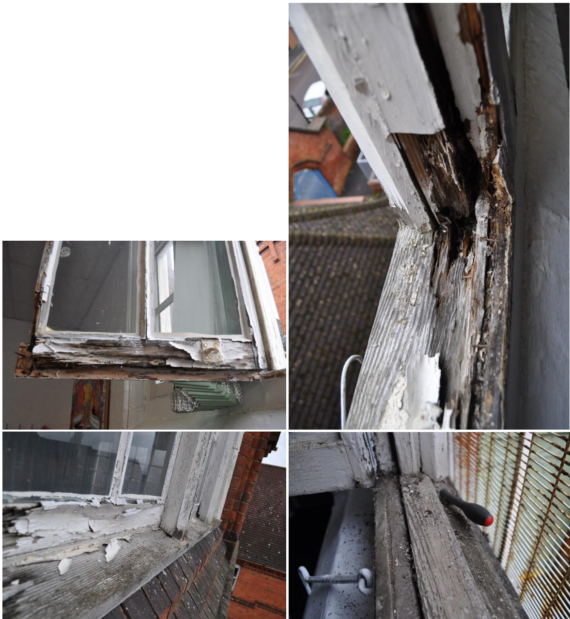
Fig 9 Examples of localized decay caused by concentration of rain water saturation in cills and at the bottom of mullions .
