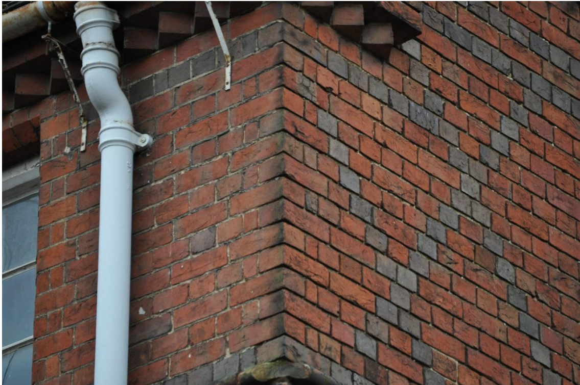
Fig 15 Showing the change from eroded west facing brickwork joints (right) to pointing surviving virtually as built on north facing brickwork (left)
