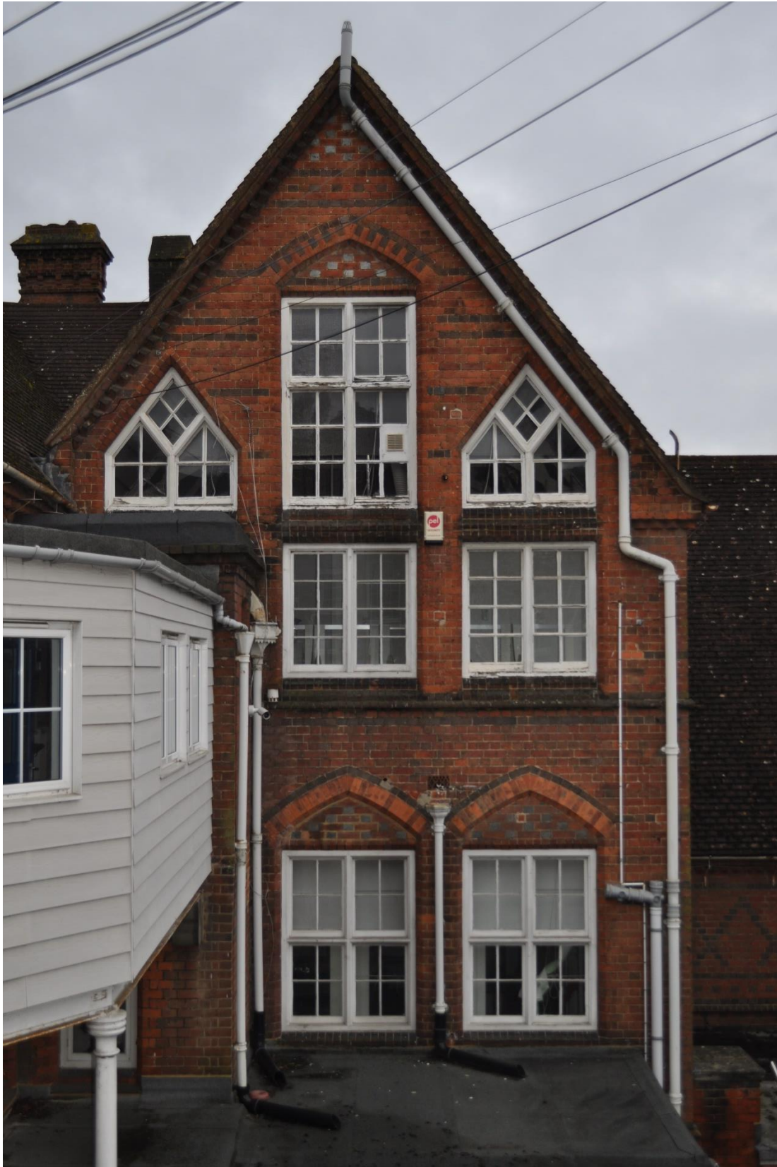
Fig 8 East elevation central wings with original timber windows, the upper parts are blocked by suspended ceilings
