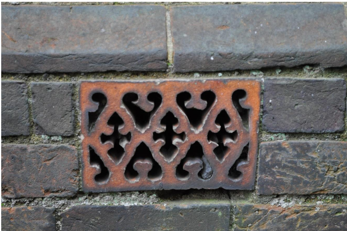
Fig 18 Standard ornamental air brick in plinth showing typical mortar loss at ground level.
