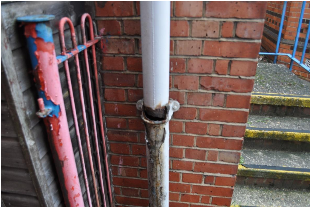
Fig 21 Broken pipe collar causing leak
