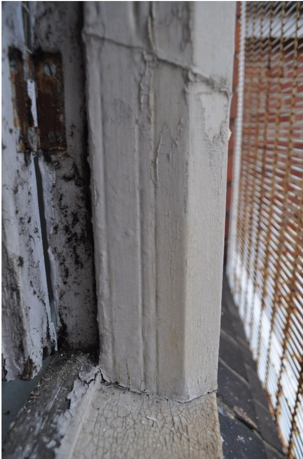
Fig 12 Example of previous scarfed in bottom of mullion
