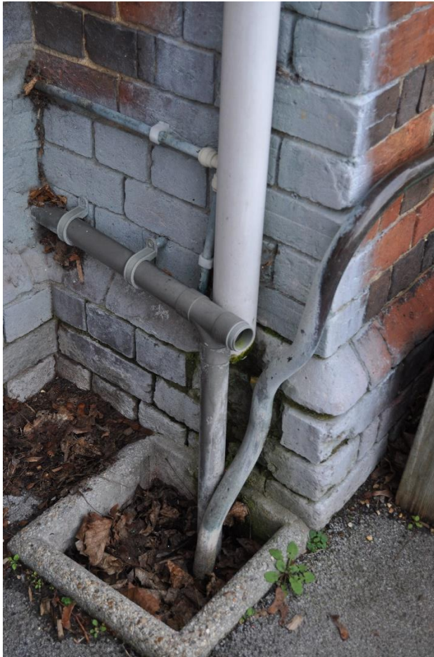
Fig 22 short down pipe and leaking services discharges causing brick damage
