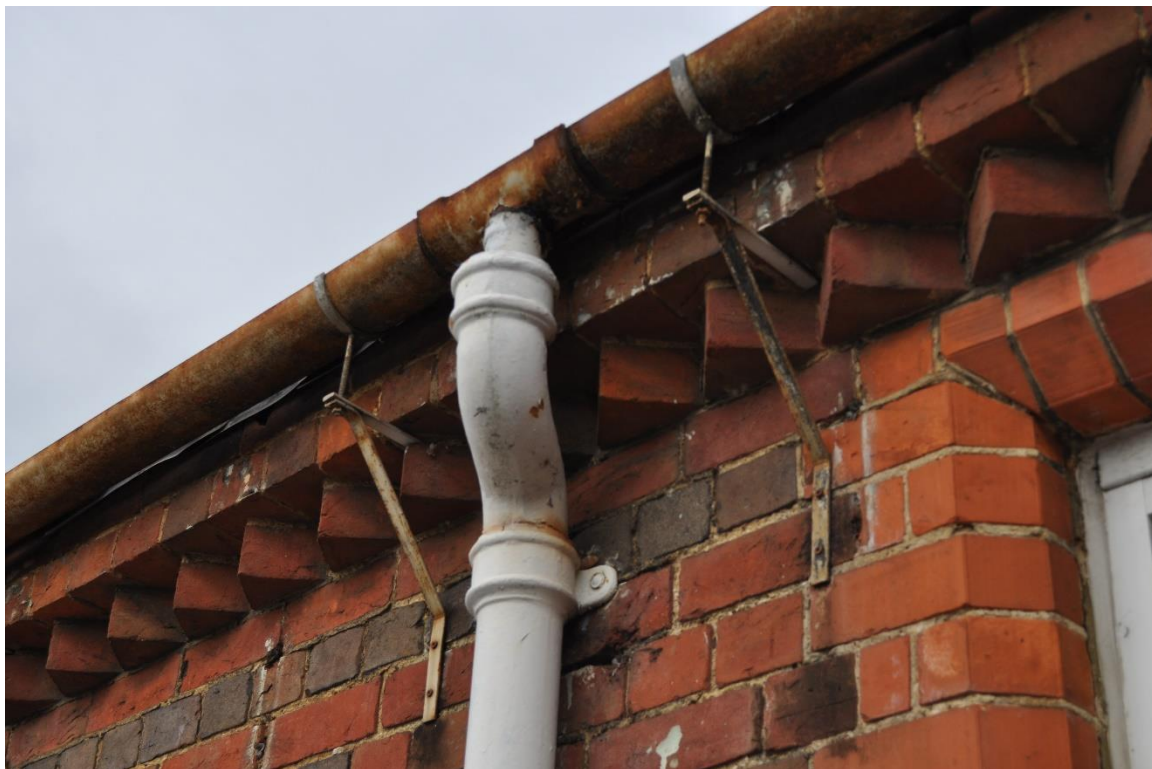
Fig 19 Corrosion of modern steel or cast gutter and steel brackets, poor connection detail at outlet
