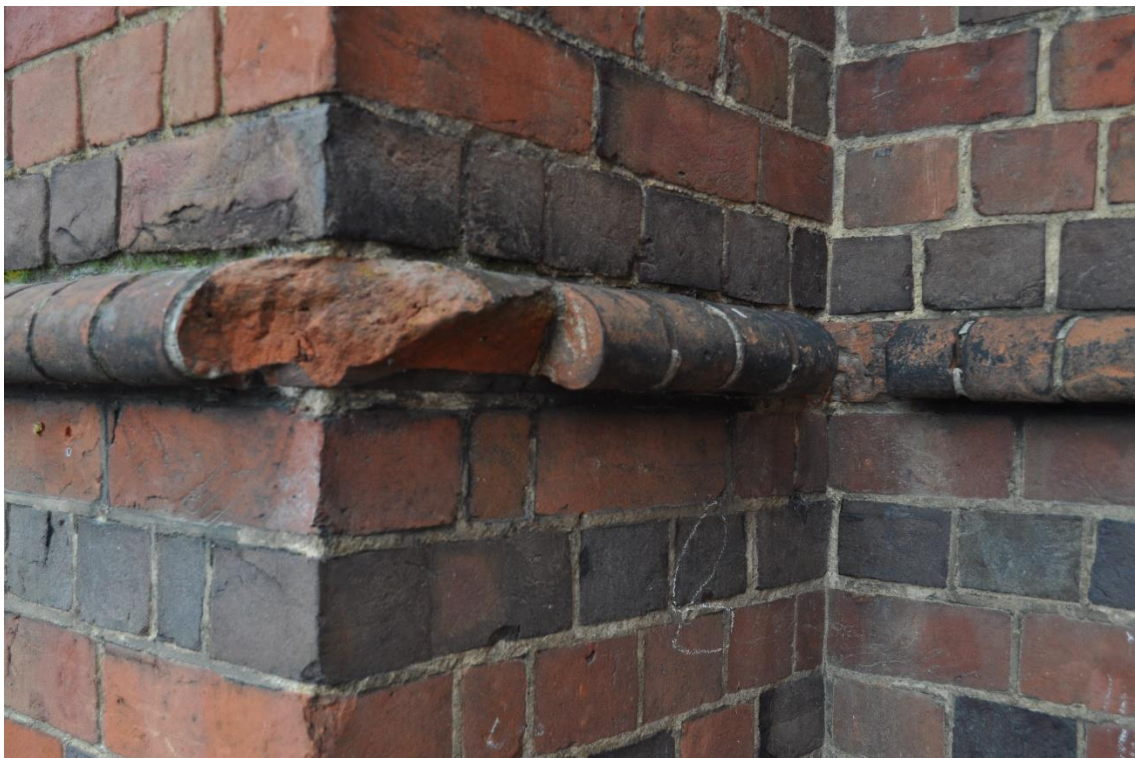
Fig 16 Example of a broken external corner string course brick.
