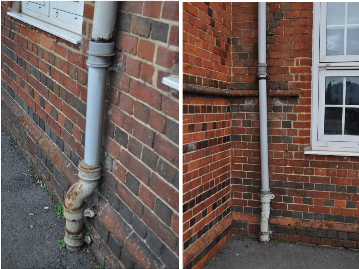
Fig 20 Examples of ad hoc repairs to cast iron using plastic, evidence of corrosion.
