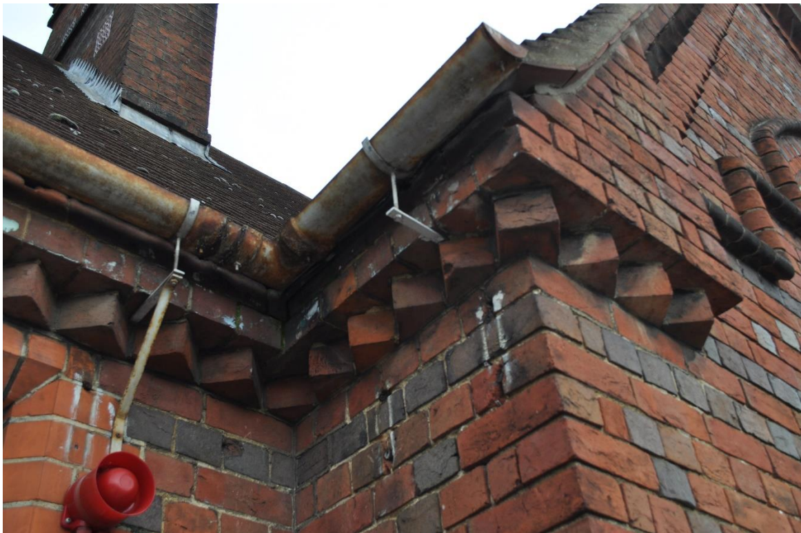
Fig 14 Open joints in high level brickwork exposed to south westerly prevailing weather
