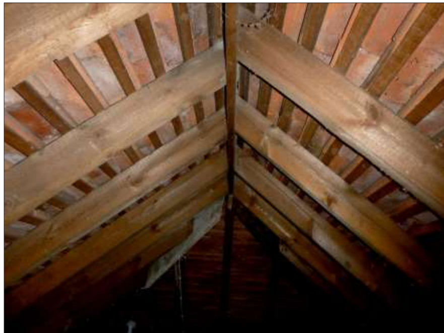
Photograph 3: Showing the unlined roof space, found to be dusty and cobwebbed throughout.
