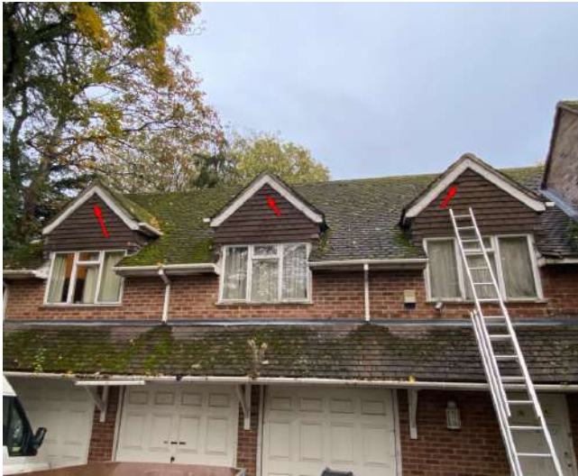
Image 1: Locations of gaps beneath hanging tiles on the western elevation
