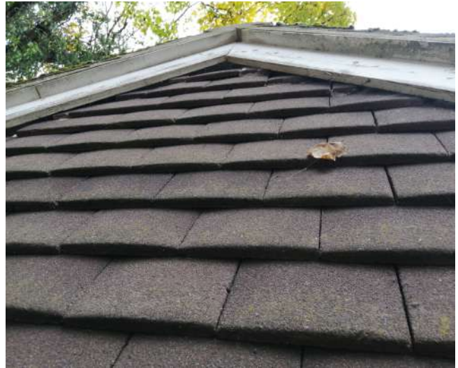
Image 8: Majority of having tiles above dormer windows well sealed, with a gap at the apex
