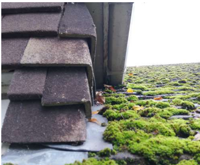
Image 9: Gaps beneath hanging corner tiles on dormer windows on the western elevation
