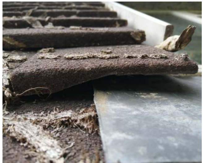
Image 16: Gap beneath hanging tiles adjacent to window on the eastern aspect of the building
