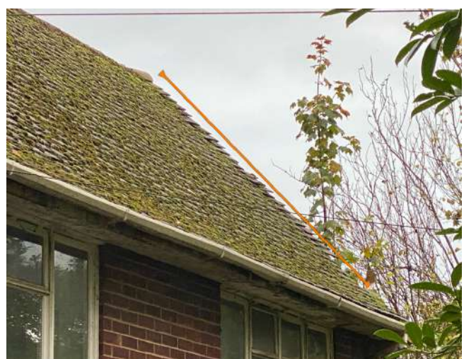
Image 6: Lifted and missing verge tiles on eastern elevation
