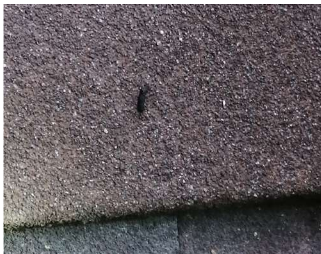
Image 17: Droppings found stuck to hanging tiles
