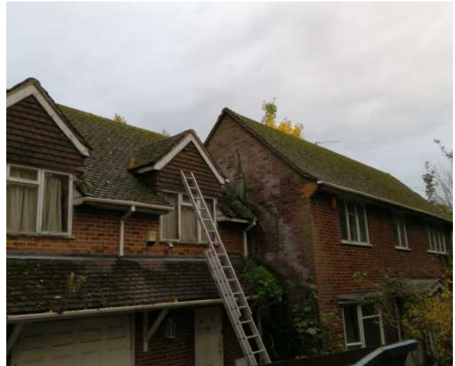
Image 2: Eastern aspect, showing coverage of moss on roof tiles
