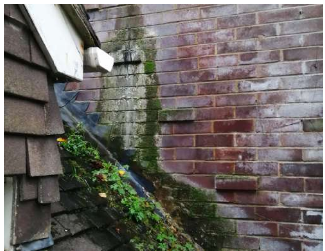
Image 12: Vegetation growing on roof tiles
