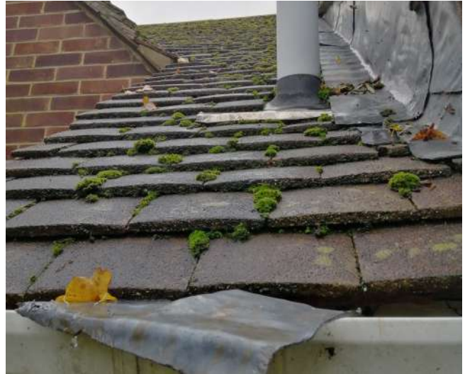
Image 14: Coverage of moss on well sealed roof tiles and lead flashing
