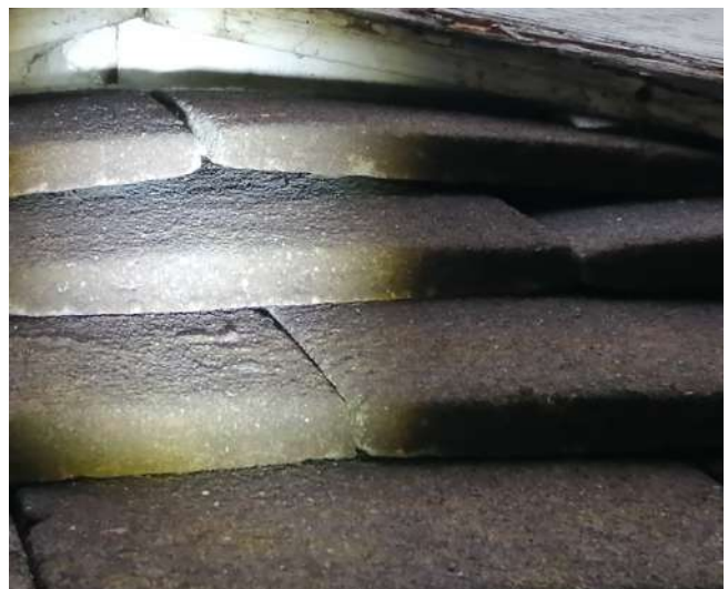
Image 10: Close inspection of gap at the apex of hanging tiles on dormer window
