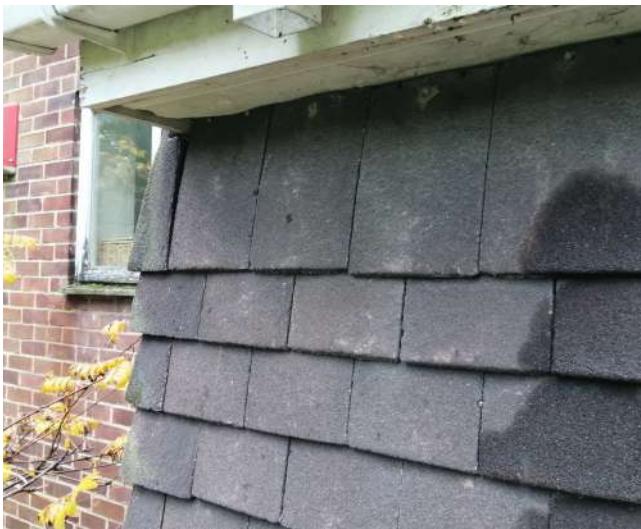
Image 15: Gap beneath corner hanging tiles
