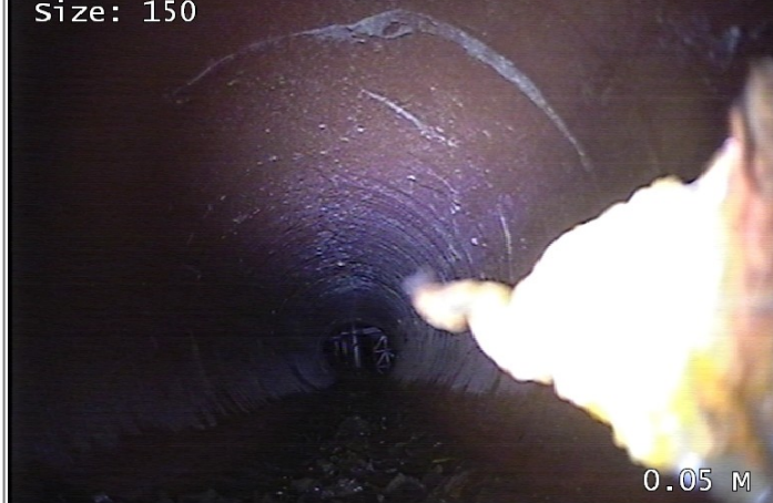
Crack longitudinal at 10 o'clock
