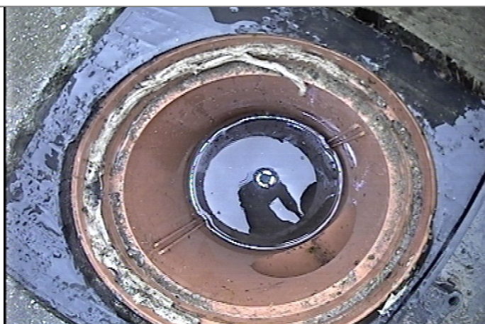
Manhole / Access Point: GULLY IN BACK GARDEN 1 Internal
