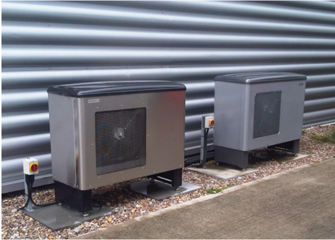
Figure 1. Air Source Heat Pumps
