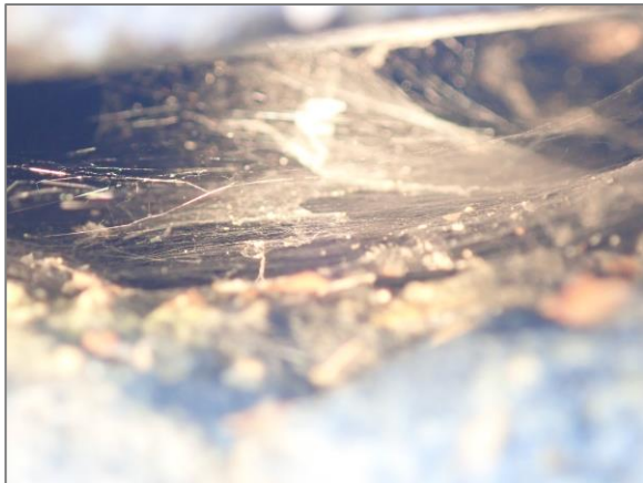
Photo 21 Cobwebs within gap
