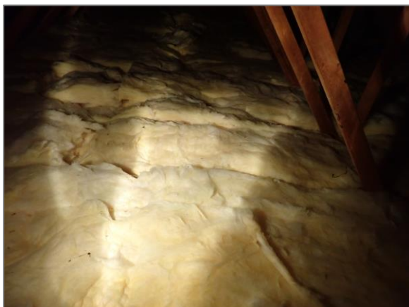
Photo 5 Loft floor insulation
