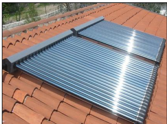
Solar Evacuated Tubes
