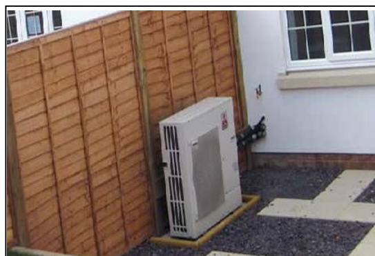
ASHP Installed on a new dwelling
