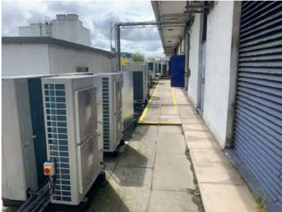
Photo 5: External area off-site on Level 2 that houses some of the building's air condition units.
