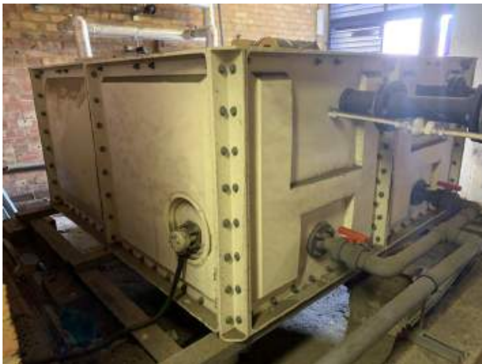
Photo 6: Water tank off-site on Level 2.
