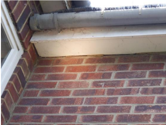
7. Missing mortar along edge of the soffit box on the rear gable end.
