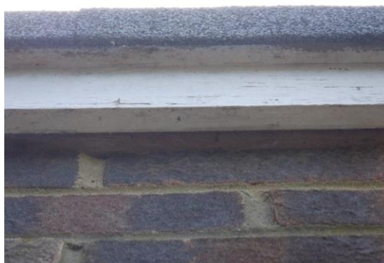
14. Bitumen felt and timber barge boards tight on the garage.
