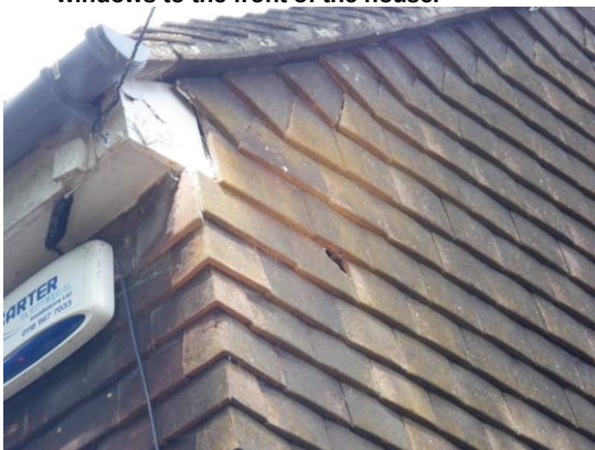
11. Broken hanging tile and gap at the edge of the soffit box at the eastern side of the house.
