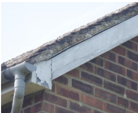
13. Gap between the timber fascia and under cloak at the rear gable end.
