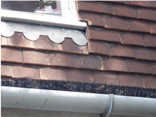
9. Gaps behind hanging tiles at the edge of the windows to the front of the house.
