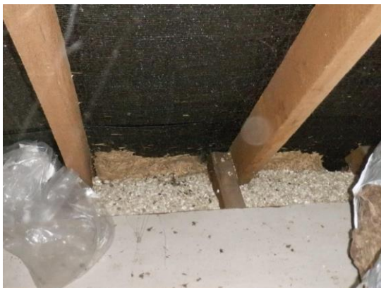
19. The eaves open in the main section of roof but old wasps' nest present.
