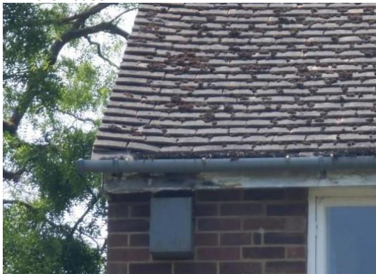
5. Roof tiles slightly lifted on the rear eastern verge.
