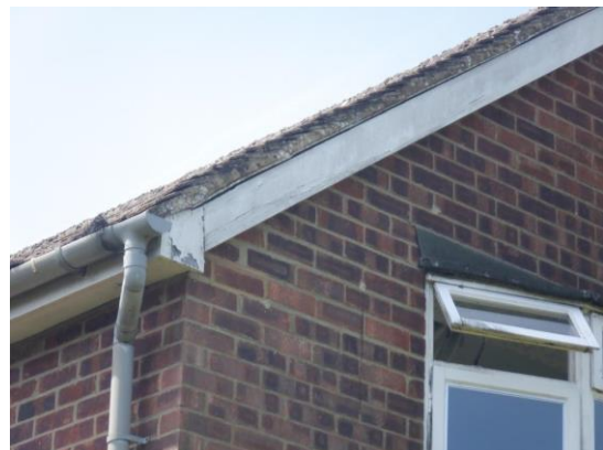
12. Verges mortared to the rear of the house.
