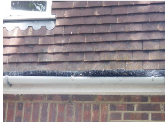
10. Lifted hanging tiles at the front of the house.
