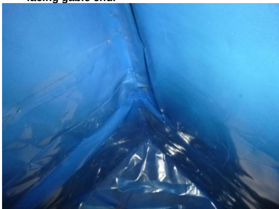
17. The unlined roof covered in plastic in eaves space 1.
