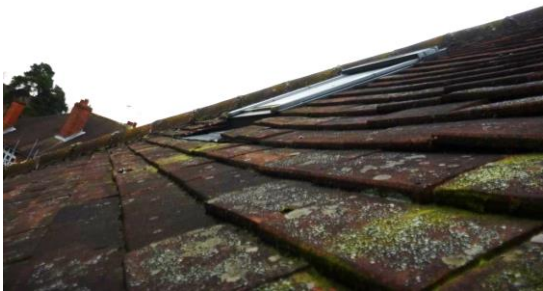
5. Gaps under the roof tiles around the skylight to the side of the house.
