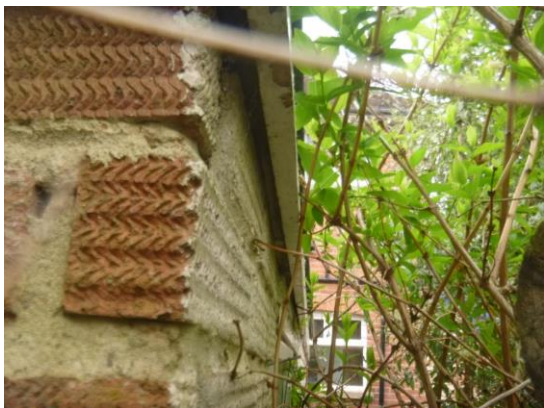
13. Small cobwebbed gap behind fascias to the rear of the garage.
