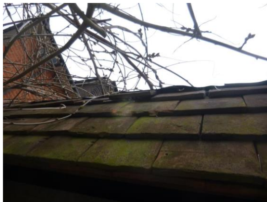
14. Strip of hanging tiles on the front of the garage lifted in places.
