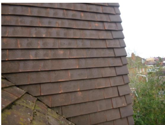
9. Hanging tiles lifted on the dormer window at the eastern side of the house.
