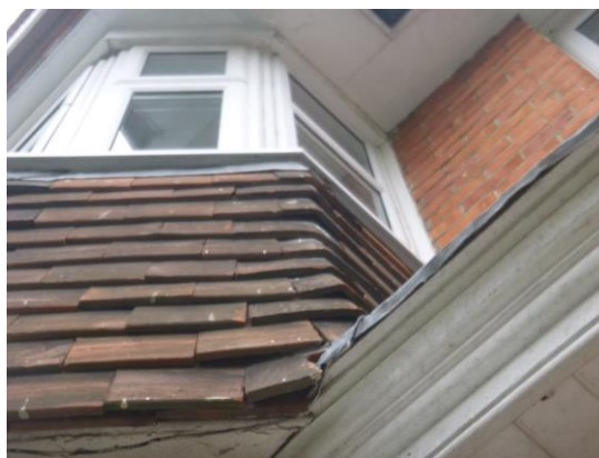
8. Corner hanging tiles lifted on the bay window to the front of the house.
