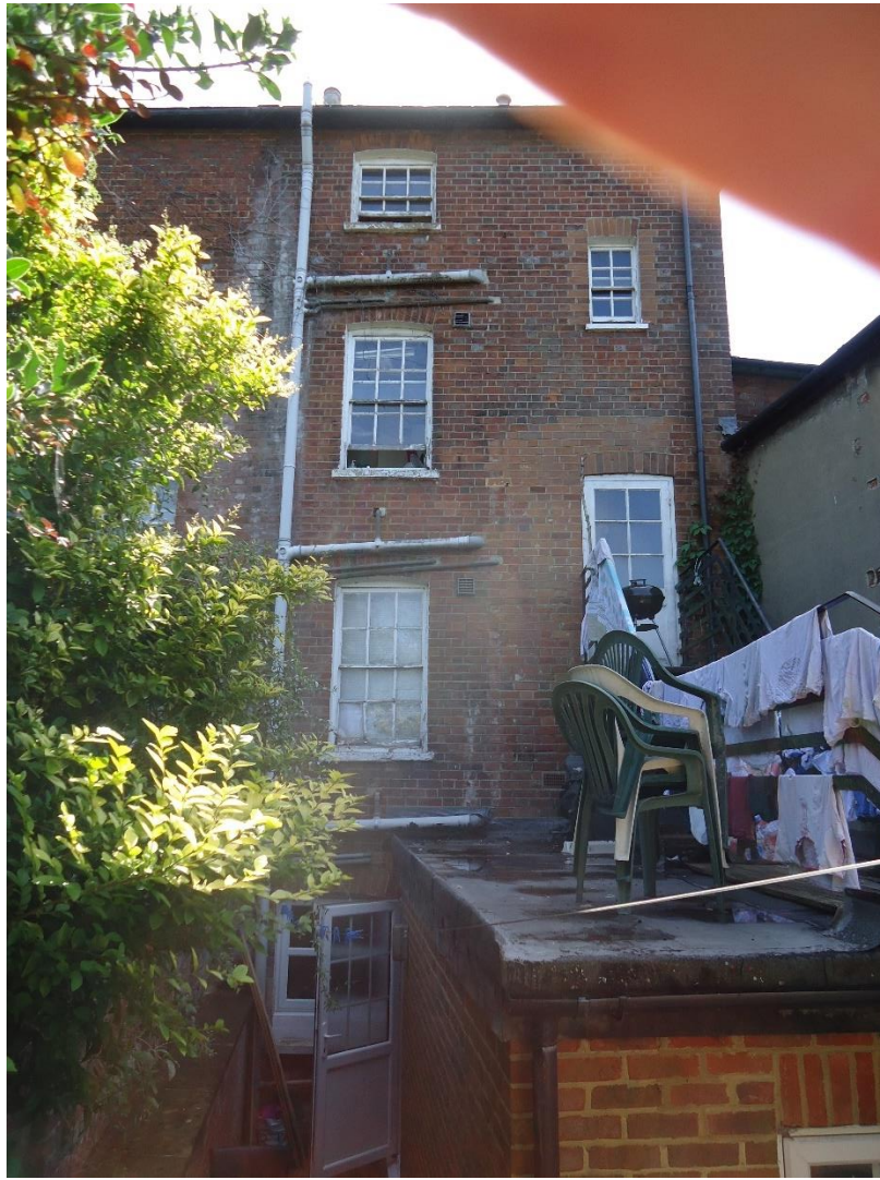
Existing dilapidated Rear to 27 Christchurch Road
