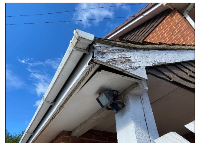
Photo 6: The hole in the soffit on the eastern elevation of B1.
