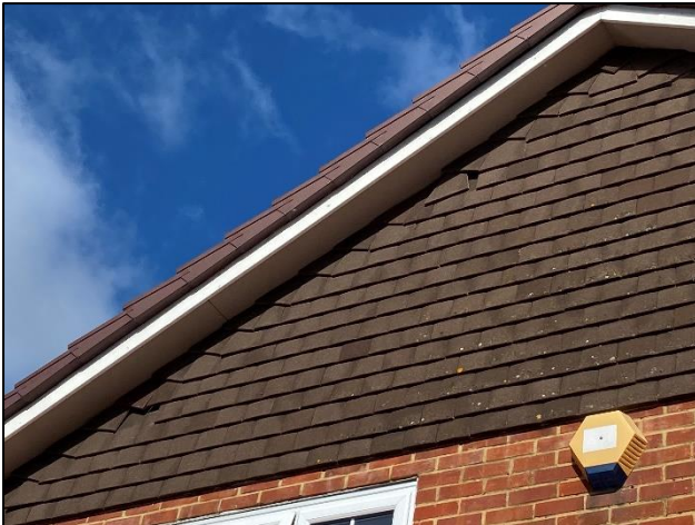
Photo 4: Examples of missing and dislodged tiles on the southern elevation of B1.
