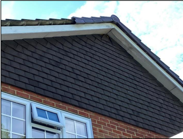
Photo 7: Broken roof protector and damaged soffit board.
