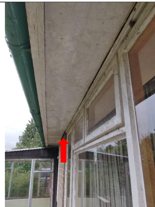
Photograph 11 – A close view of the soffit box on the east aspect. Note small gaps between the soffit and wall.
