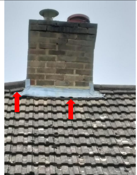
Photograph 9 – A close view of the chimney stack. Note that the chimney stack is leaning and there are gaps underneath lifted tiles and lead flashing.
