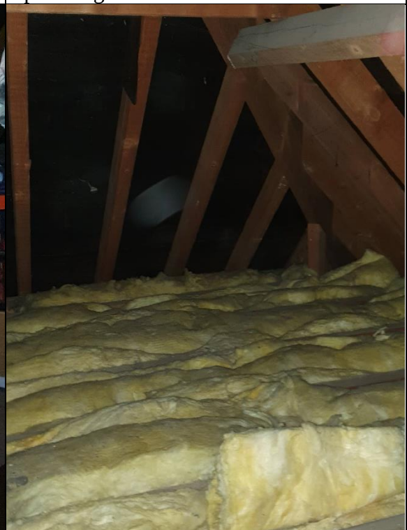
Photograph 12: Insulation lifted to check for droppings.
