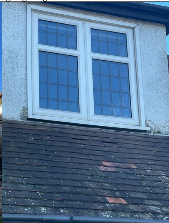
Photograph 8: Minor lifting in tiles on front porch (area not affected by works).
