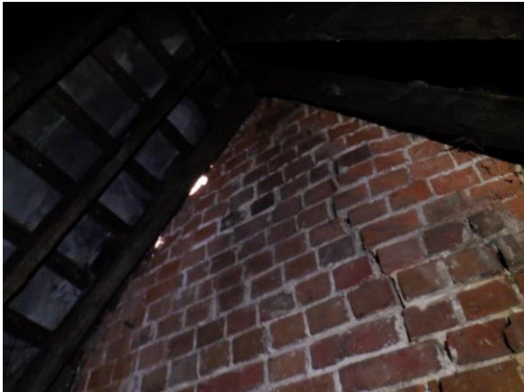
27. Daylight visible at north-eastern gable end.
