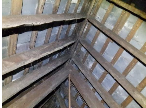
26. Daylight visible along ridge.
