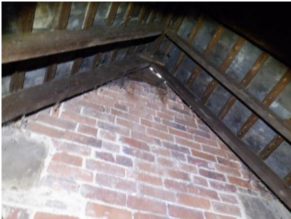
29. Daylight visible at gable apex.
