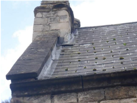
19. Lifted lead flashing at north-eastern gable end (northern elevation).
