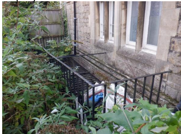
12. Overgrown vegetation at the rear of the house (TN1).
