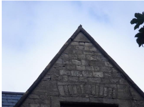
20. Recessed masonry mortar (southern elevation).
