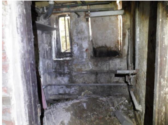
38. Gaps through windows.
