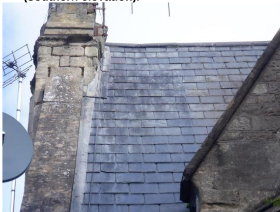
18. Missing mortar beneath ridge tiles (southern elevation).
