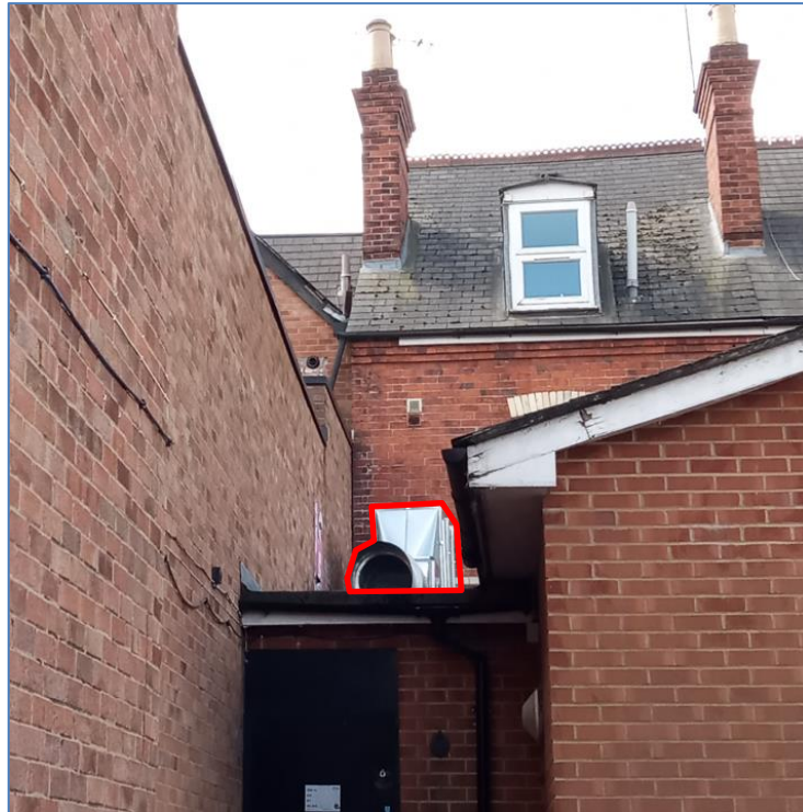
Fig 3. Rear of 734-736 Oxford Road. Ventilation and extraction equipment outlined in red. Photo taken by case officer on 01/04/2022.
