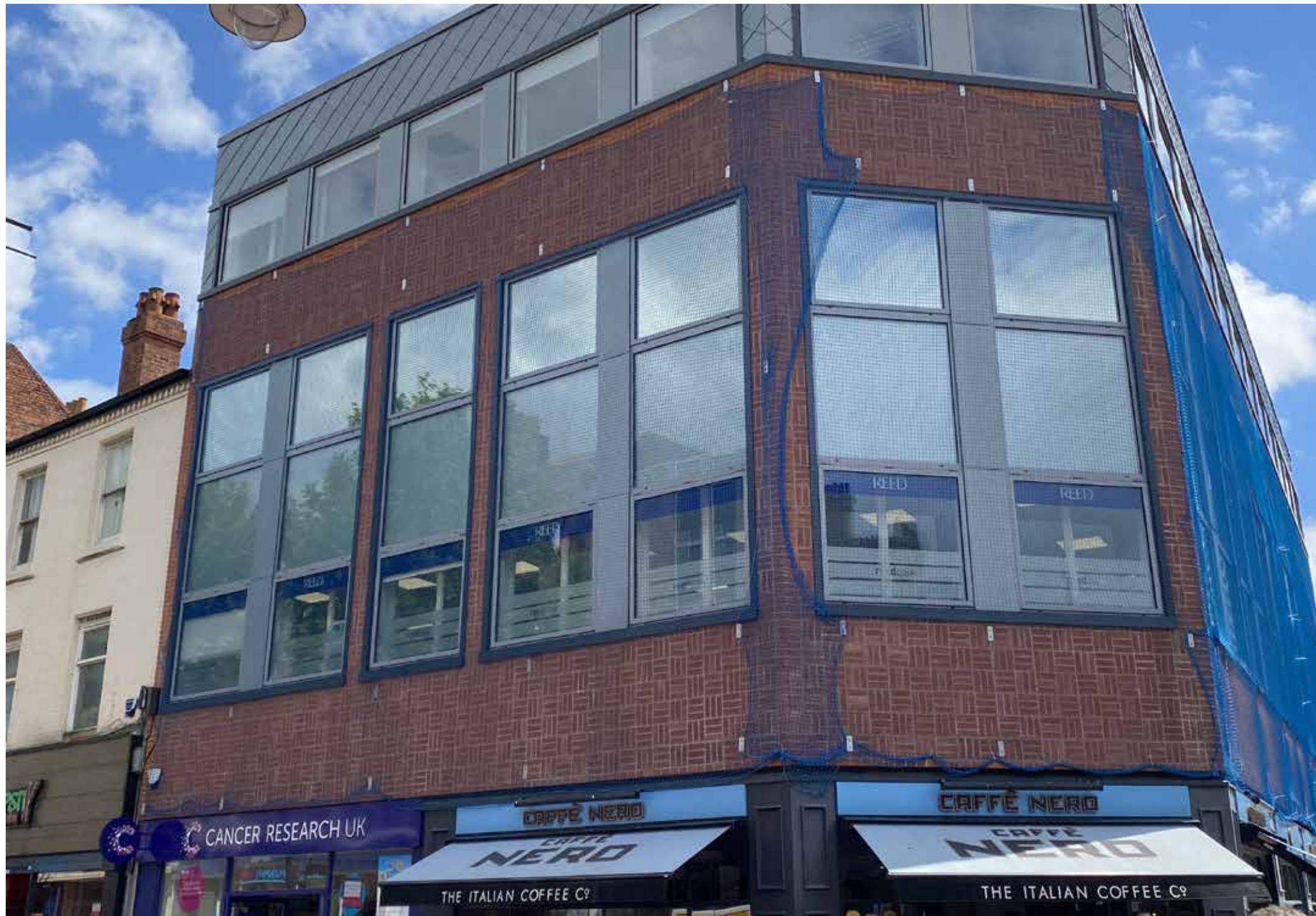
Figure 1 St Mary's House, June 2021, showing safety netting over brick slip cladding
