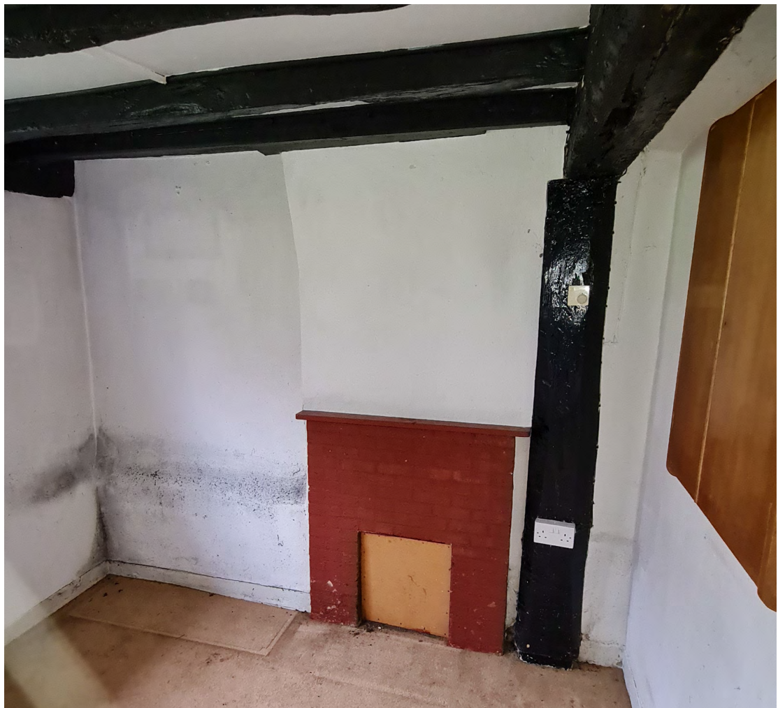
Fig 15: Internal view of the Dining Room and South-Western fireplace. Note damp to wall on left-hand side.
