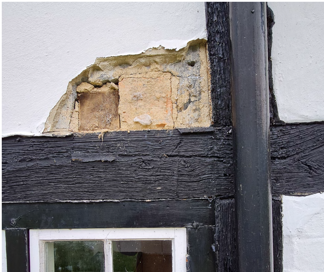
Fig 9: Section of blown render to the South-East elevation. Note modern masonry infill and the end of the first-floor joist behind.
