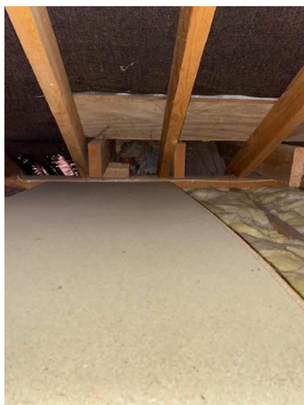
Visible light and small gap leading to adjoining roof space in eastern loft
