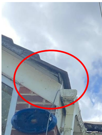
Missing cement within front elevation
