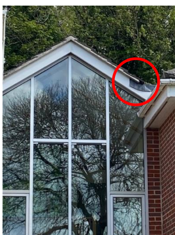
Missing cement in tile adjacent to flashing in rear elevation
