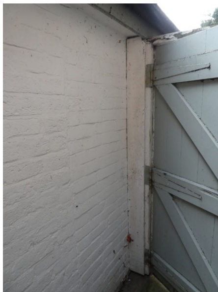
Figure 19: Blocked door opening on the left hand side of the north-west elevation
