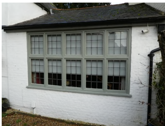
Figure 14: Change from stretcher bond to header bond on the left hand side of the 1920s window
