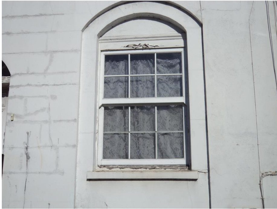
Figure 5: Present day window replacement, with incorrect glazing bars.
