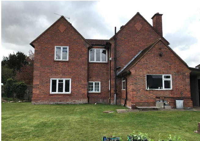
Rear elevation showing a loss of symmetry
