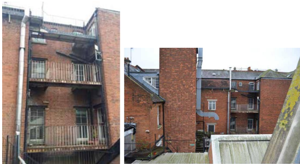
Figures 22 and 23: Poor quality rear elevations of the site
