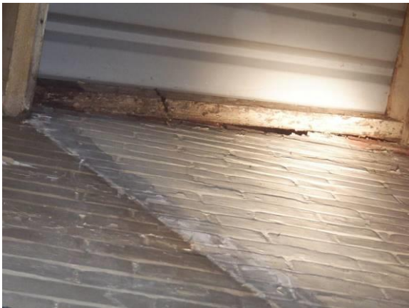
15. Slight gap between brickwork and metal rafters at the western gable (B1)
