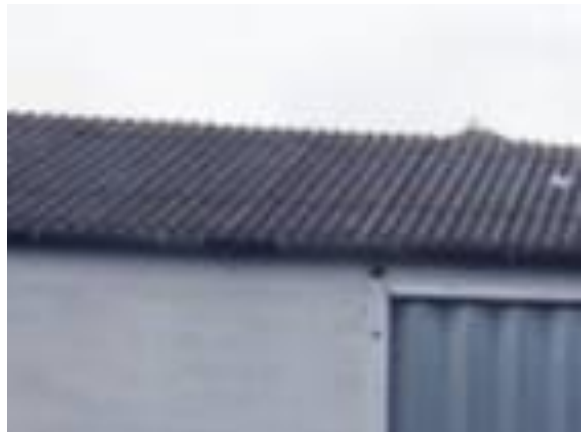
24. Corrugated asbestos roof on warehouse (B3).
