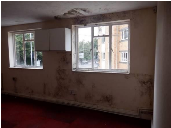
23. Water damage and damp in internal of the office (B2)
