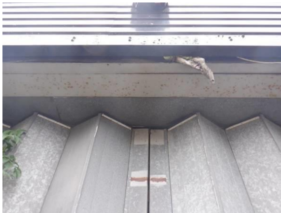
12. Metal shutters tight to the framework on the double door, northern elevation (B1)
