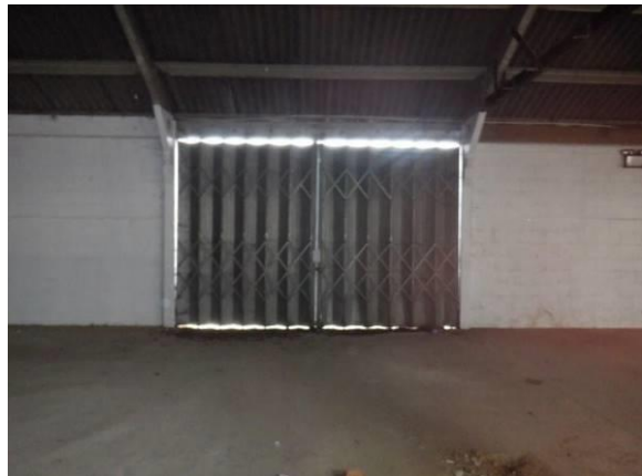
30. Daylight visible over the top of the metal double doors
