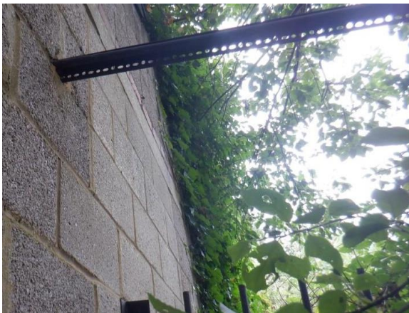
27. Ivy growing up the north-western corner of the warehouse (B3)
