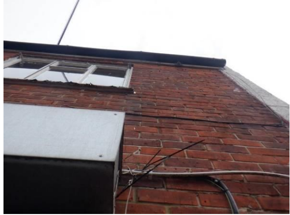
20. Slight gap below barge board along western elevation (B2)
