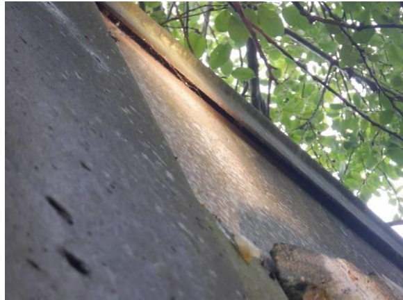
26. Gap under asbestos sheets at the northern gable of the warehouse (B3)
