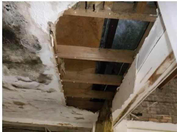
16. Broken sections of false ceiling in eastern side of the building (B1).
