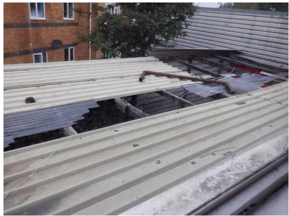
22. Broken corrugated metal and plastic roofing sheets on storage yard (B2)
