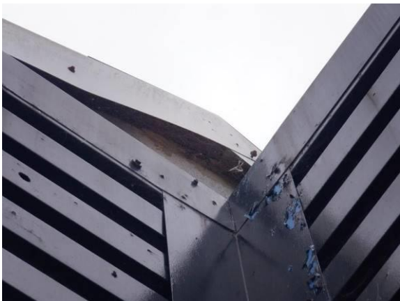
11. Slight gap behind fascia on the eastern gable of the warehouse (B1)
