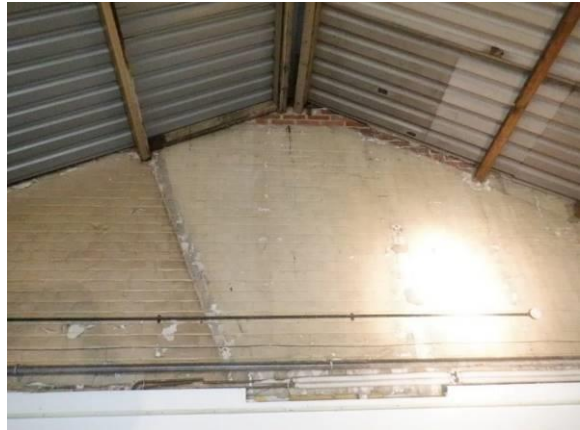
14. Brickwork tight to rafters at the eastern gable (B1)
