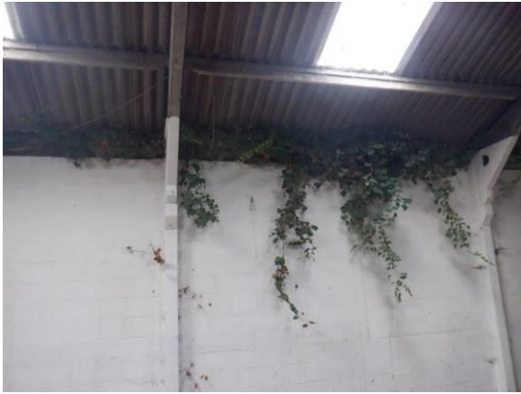
31. Ivy growing over the top of the wall plate (B3)
