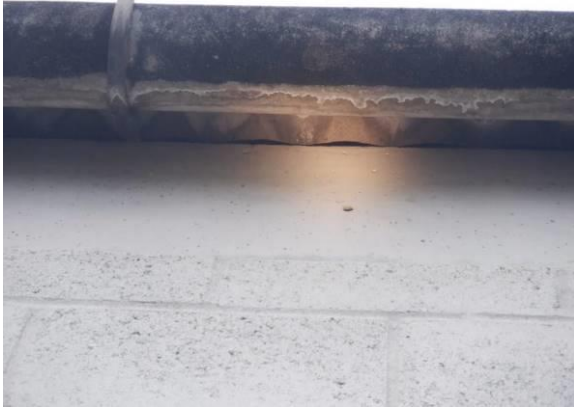
25. Small gap above the blockwork, behind the gutter on the eastern elevation (B3).
