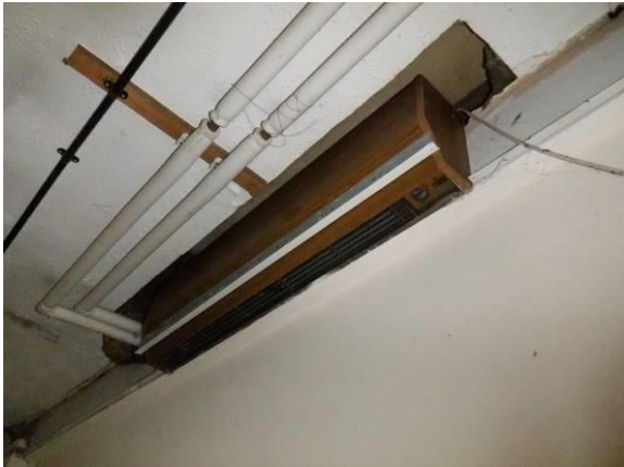
17. Asbestos roofing visible above aircon unit (B1)
