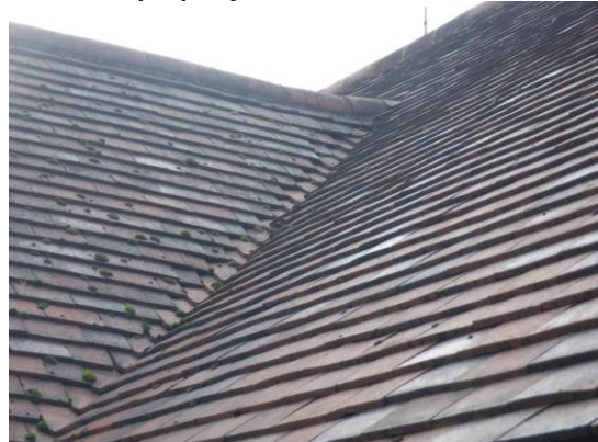
4. Gaps under roof tiles along roof valley (front elevation).
