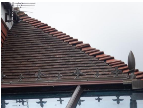
7. Mortar absent beneath hip tiles (rear elevation).
