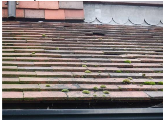
6. Gaps under roof tiles below dormer window (rear elevation).
