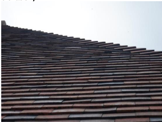
5. Gaps under roof tiles near roof hip (front elevation).
