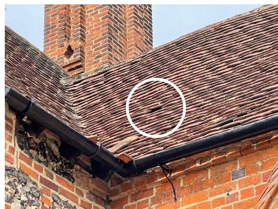
Missing tile on southern aspect.
