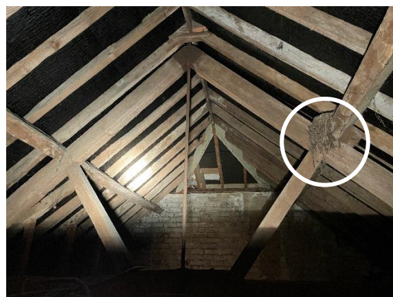
Bird nest within the western loft space of the garage.
