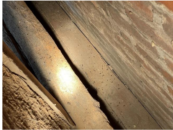
Accumulation of droppings below central ridge beam.
