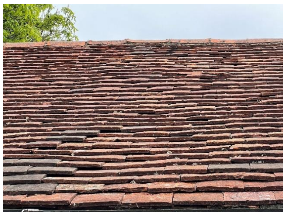
Naturally occurring gaps under roofing tiles on western aspect.
