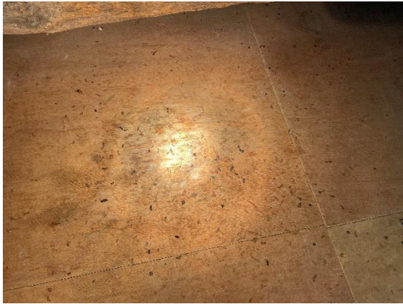
Accumulation of droppings below northern ridge beam.
