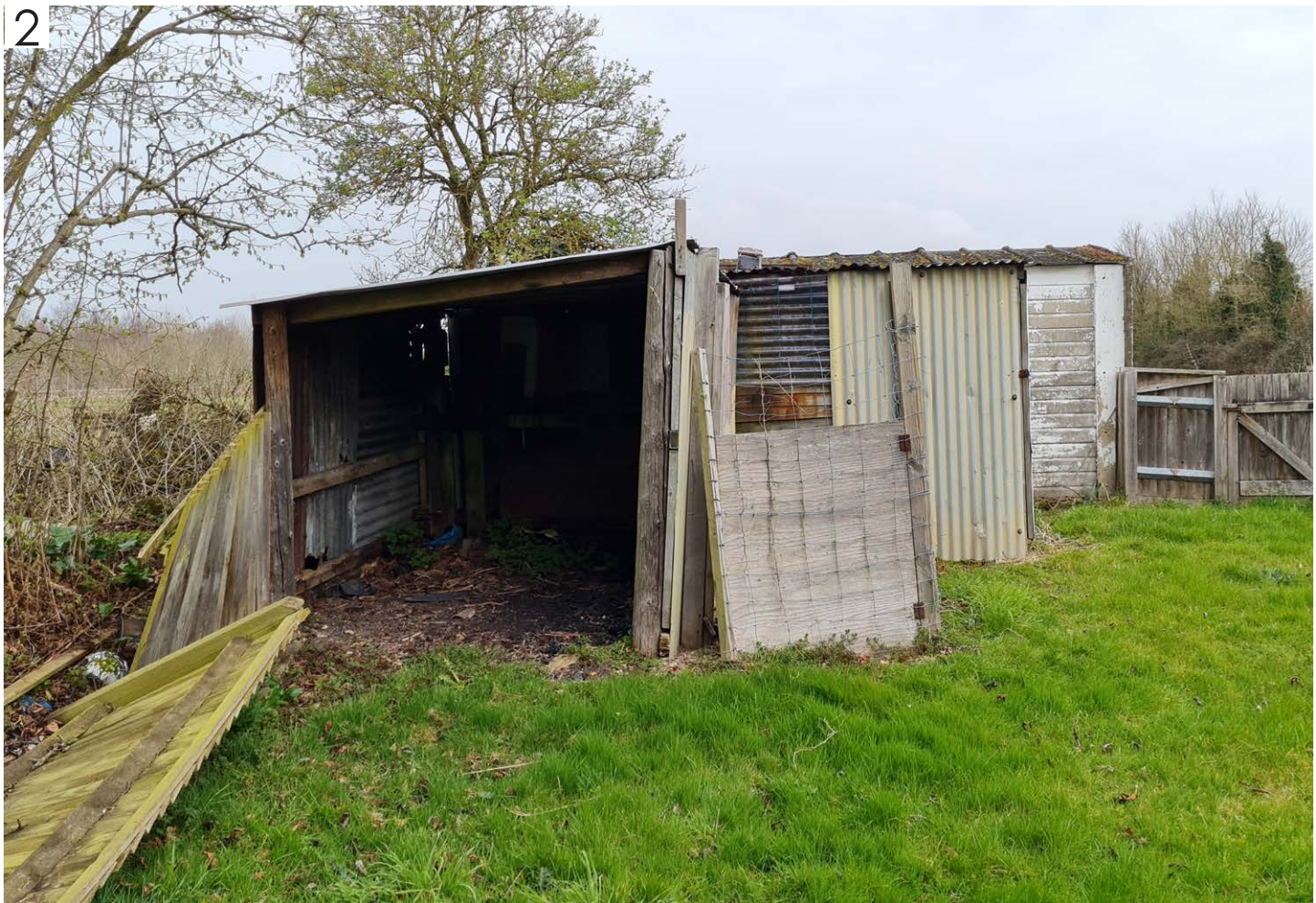
View of side of concrete garage and open end of dilapidated storage structure, looking North.
