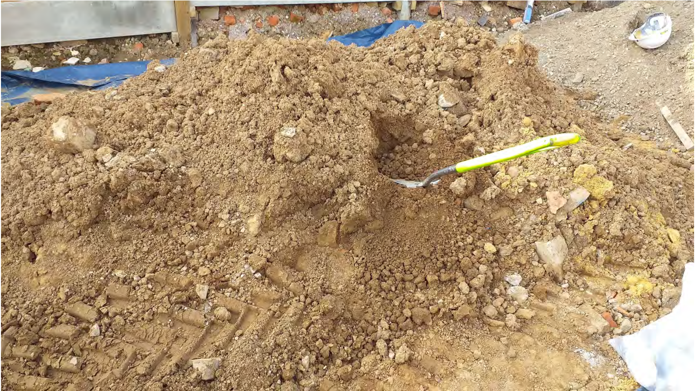
The stockpiled soil from the over excavated oil spillage area
