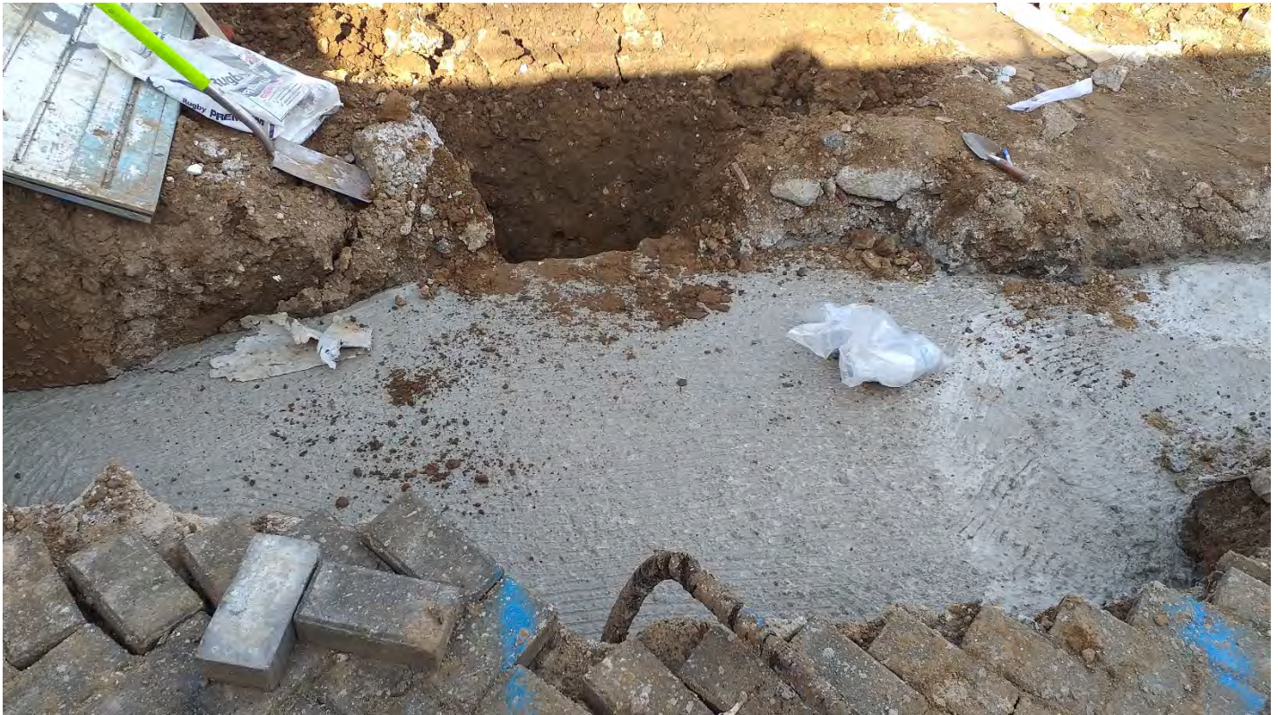
Above, the over excavated foundation in the borehole BH8 area
