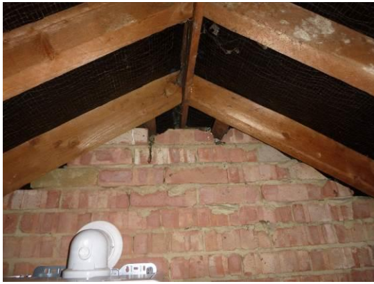
25. Large gap at the apex of the southern gable end.
