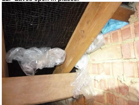
24. Gaps filled with plastic at the edges of the brickwork at the southern gable end.
