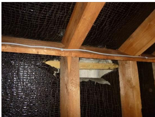
16. Large tear in roof felt.
