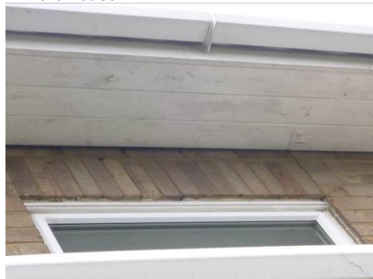
12. Gap behind the soffit box to the front of the house.
