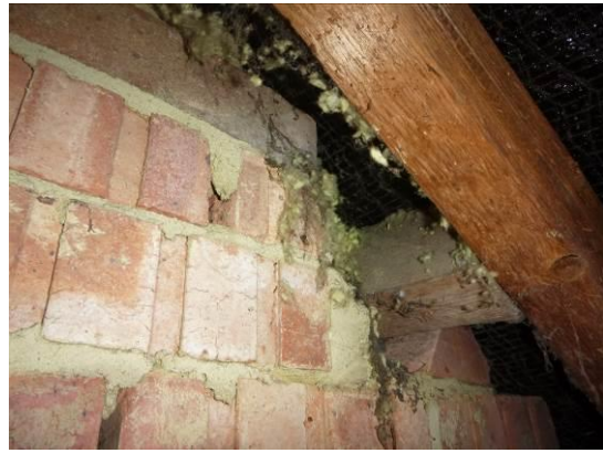
26. Shredded fibreglass visible in the southern gable end.
