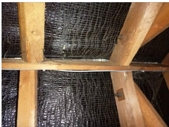
19. Roofing felt loose along the ridge.
