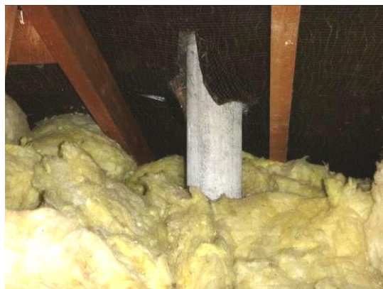
20. Roofing felt loose around the flue pipe.
