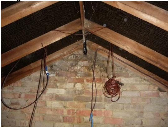
27. Gaps between the end rafter and brickwork at the northern gable end.
