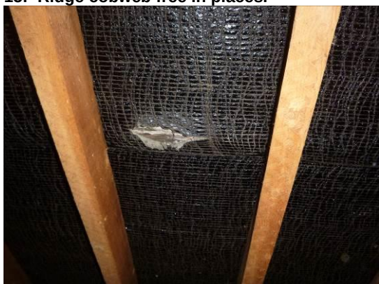
17. Large tear in roof felt.
