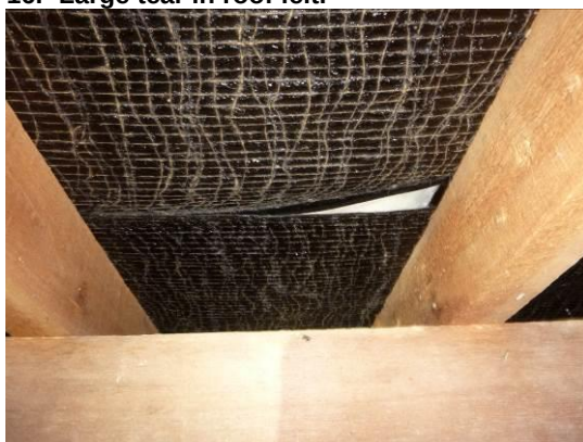
18. Roof tiles exposed where the sheets of felt overlapped.
