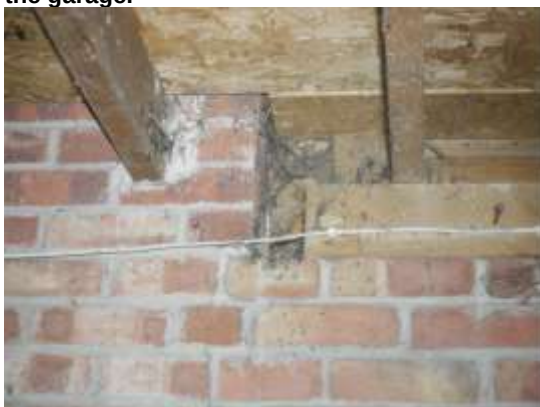
25. Daylight between soffit and wall of garage and house.
