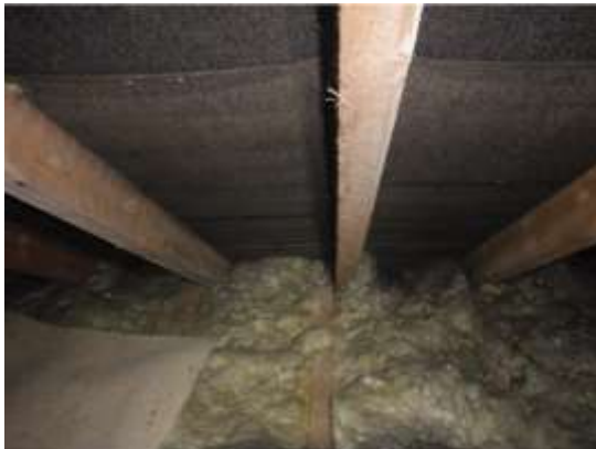
21. Some eaves left open whilst others filled with fibreglass insulation.
