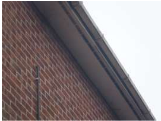
8. UPVC soffit tight to the brick wall, viewed from the north.
