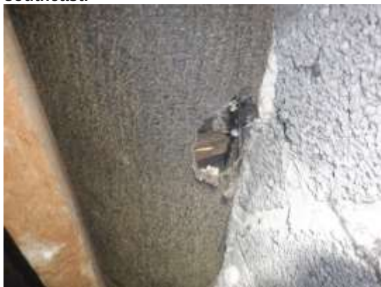
17. Small tear in bitumen felt.
