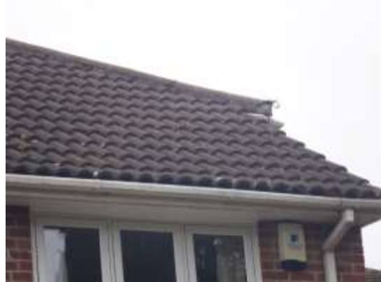
4. Fully mortared hips viewed from the southwest.
