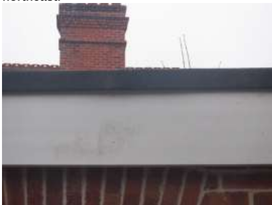
11. Felt tight to the UPVC soffit, viewed from the southwest.
