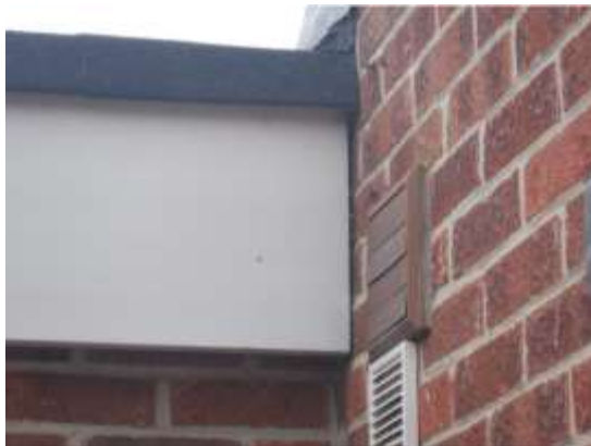
15. UPVC Soffit not fully attached to brick wall of the main property, viewed from the southeast.
