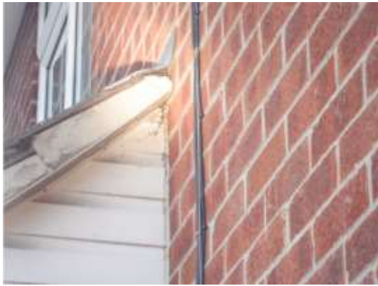
7. Lifted lead flashing with brick wall visible behind, viewed from the northwest.
