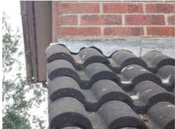
6. Lifted lead flashing with brick wall visible behind, viewed from the northeast.
