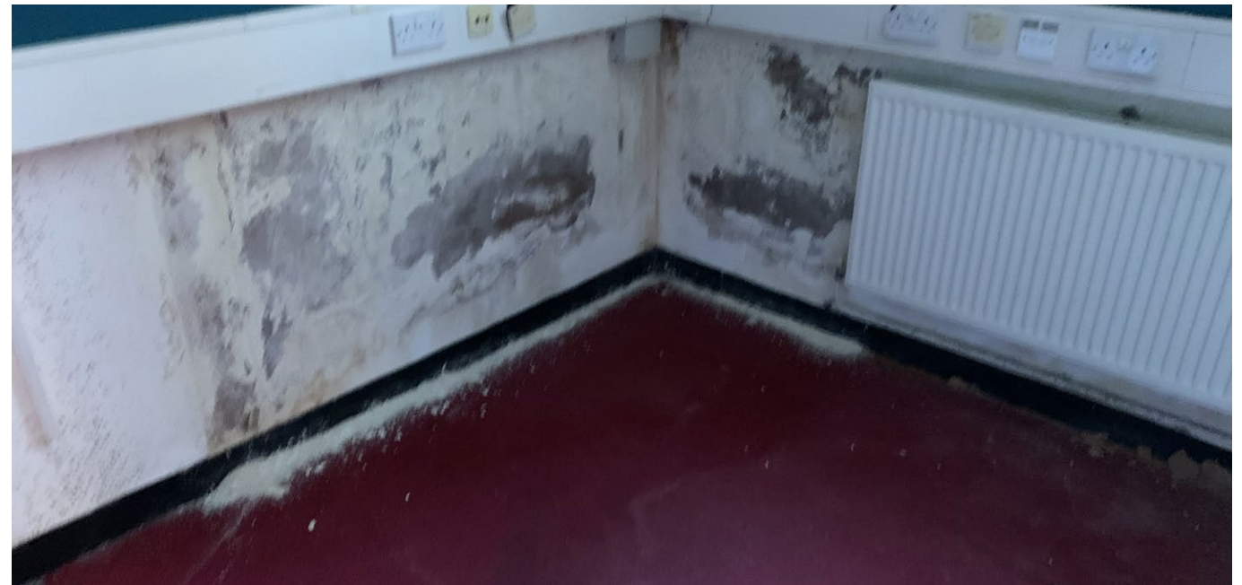
Area awaiting scheduled repairs
