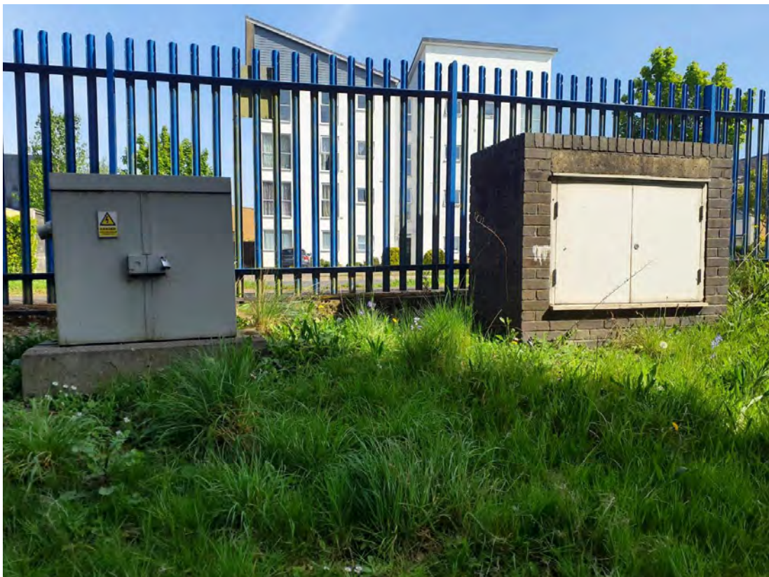
Plate 32 - Electrical service boxes located in the north-western corner of the site.
