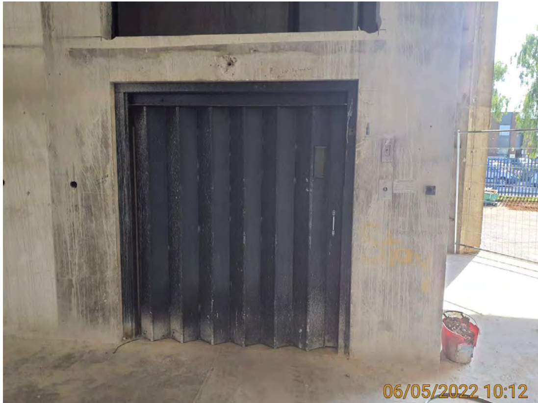
Plate 15 - Goods lift adjacent to central Eastern stairwell.
