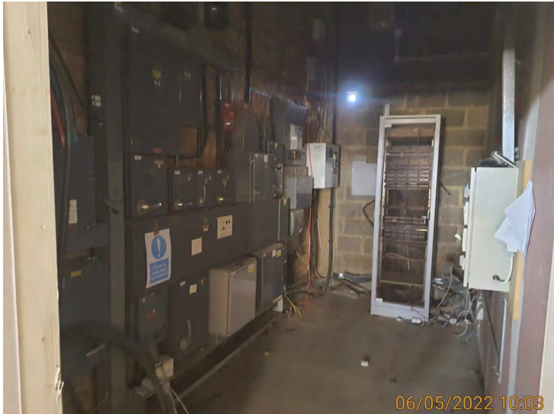
Plate 5 - Fuse box and server room.
