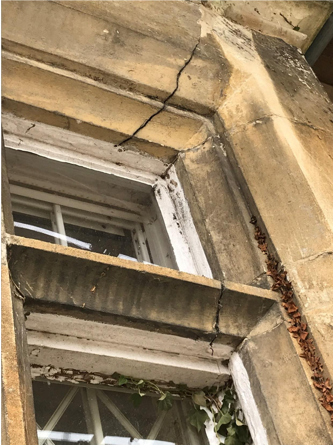
Example of cracking to transom and window head
