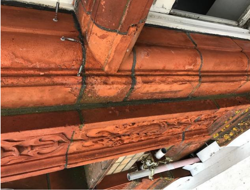
Cement pointing causing failure of the terracotta.
