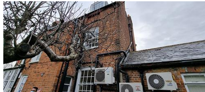
Existing air conditioning units
