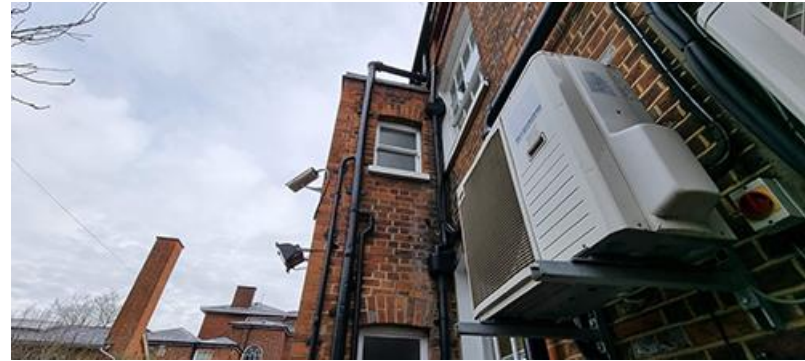
Existing soil & Vent pipe
