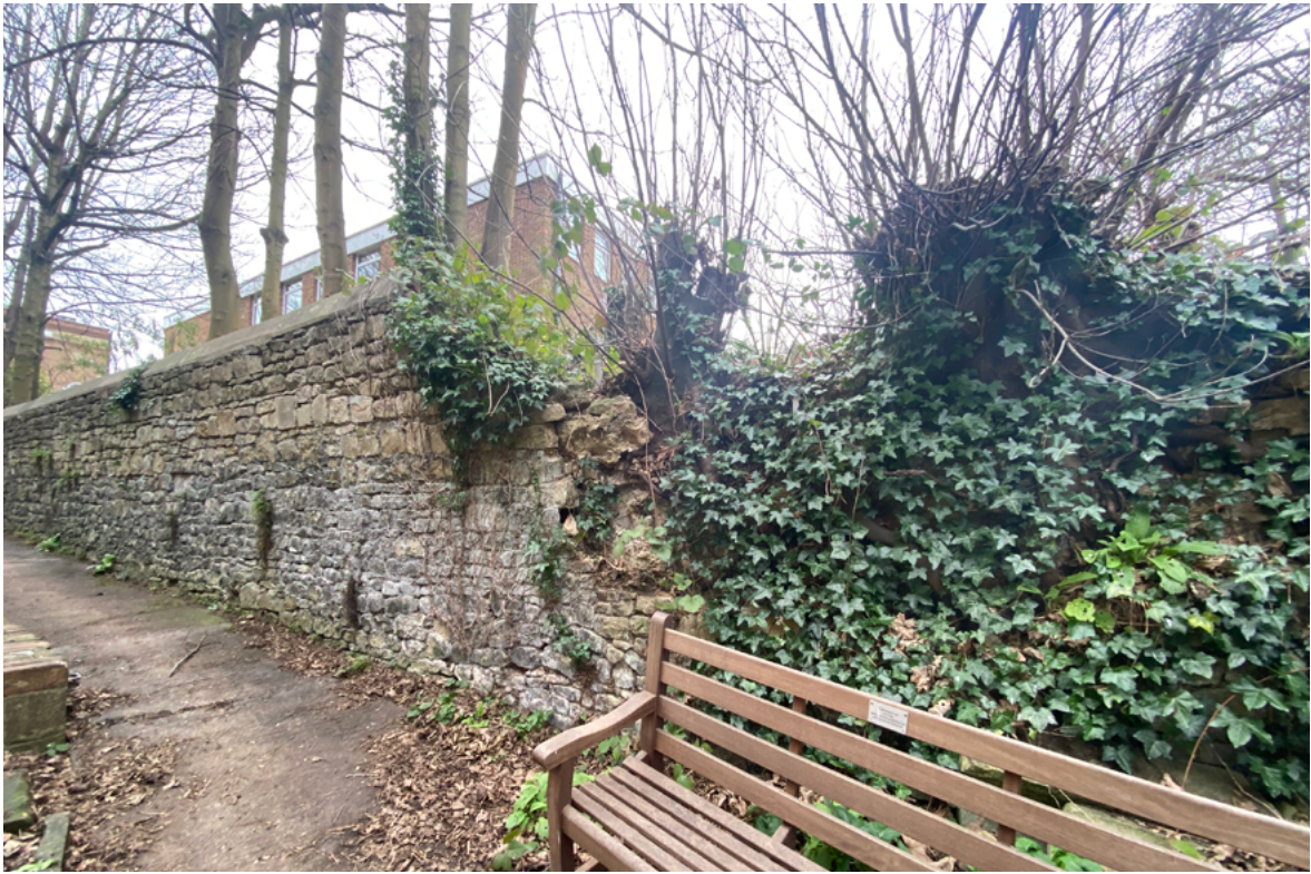
Fig.5: View of self-seeded sycamore trees causing partial collapse to boundary retaining wall
