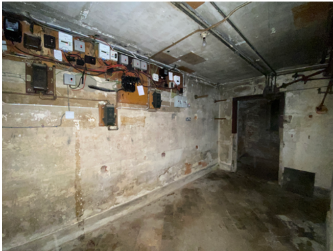
Fig. 13-15: Photographs of building dilapidations
