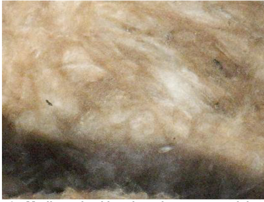
19. Medium-sized bat droppings on top of the new layer of fibreglass insulation (front side of the roof void).
