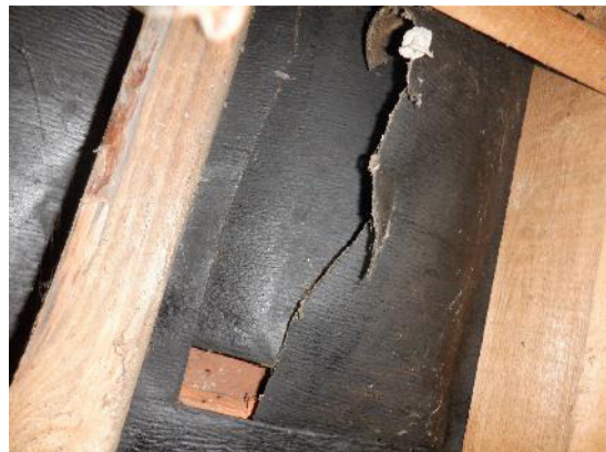
12. Tear in roofing felt.
