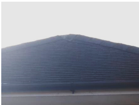
3. Lifted roof tiles (front elevation).
