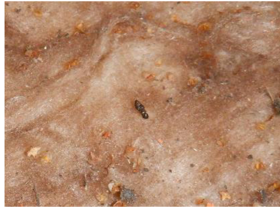
16. Small-sized bat dropping below gap in roofing felt.
