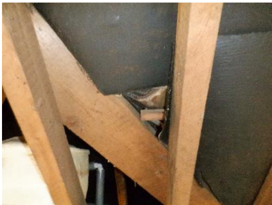
11. Gap in bituminous roofing felt (rear elevation).
