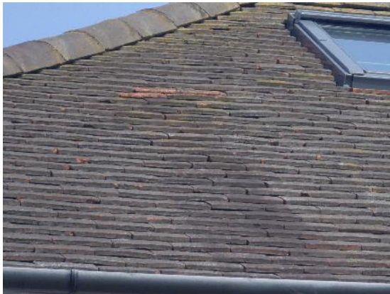
5. Lifted roof tiles beside rooflights.
