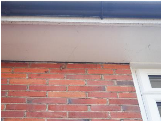
9. Gap between the soffit and brickwork (rear elevation).
