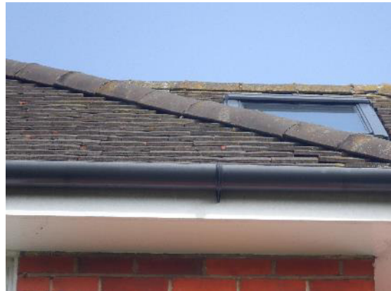
6. Gaps below hip tiles.
