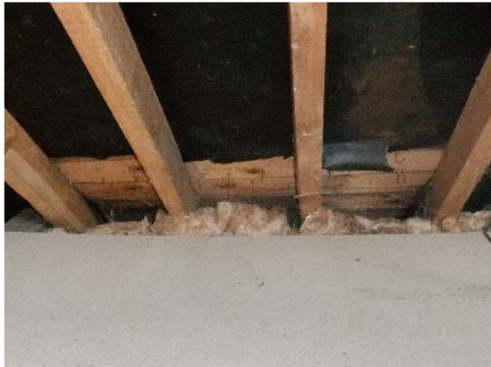
15. Boarding along the eaves on the southern elevation.
