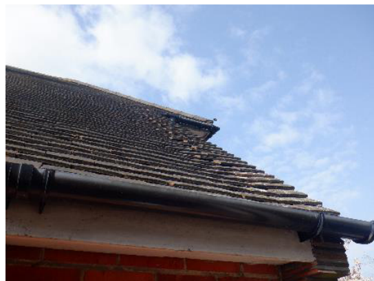
4. Lifted verge roof tiles (southern elevation).
