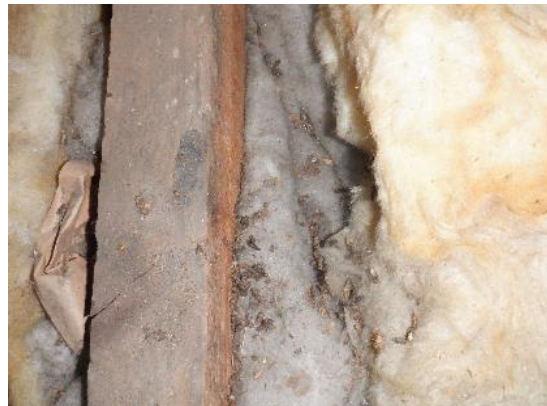
18. Pile of medium-sized bat droppings on top of old layer of fibreglass insulation
