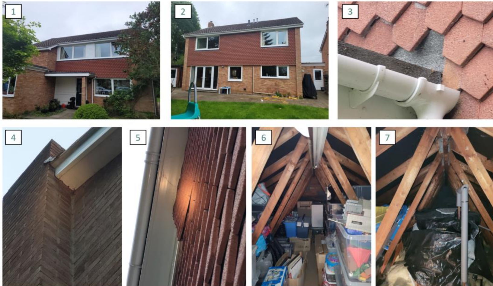
1: Front view of the house. 2: Rear view of the house. 3: Example of a gap under the hanging tiles. 4: Gap where soffit meets the chimney 5: More gaps at the hanging tiles 6: Loft view facing east 7: Loft view facing west
