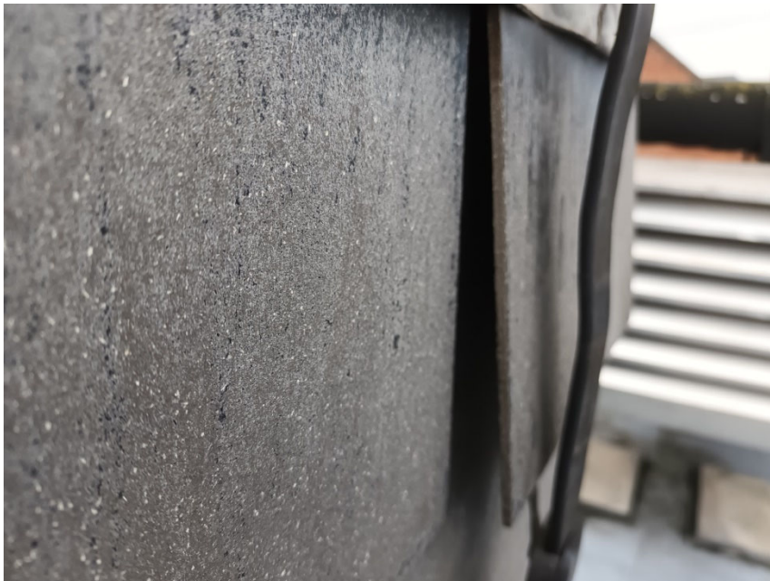
Photo 2. Lifted exterior tile
