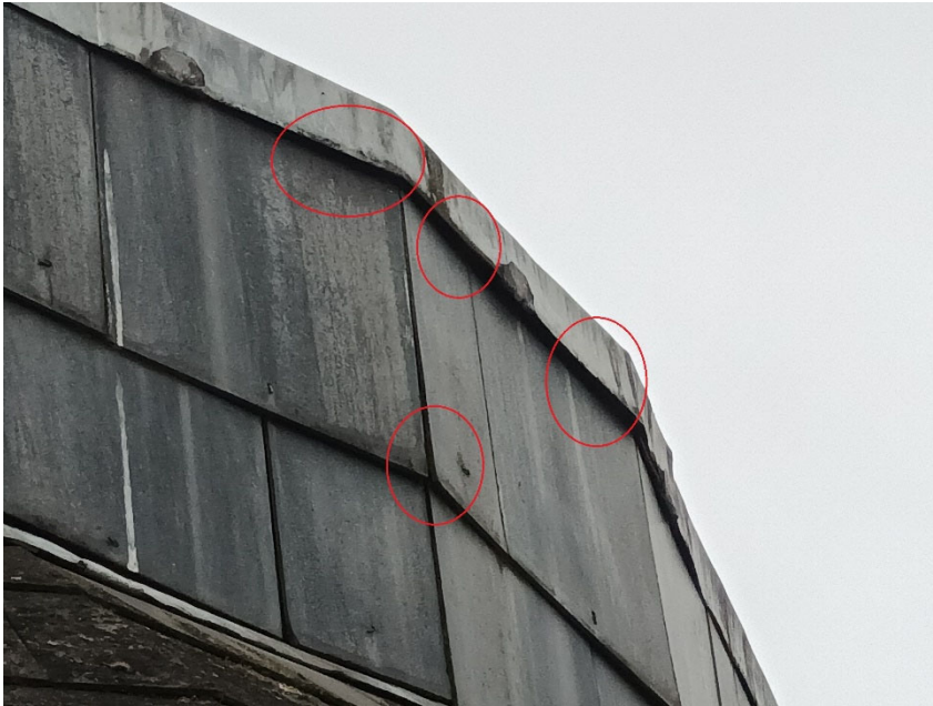
Photo 5. Lifted lead flashing and tiles
