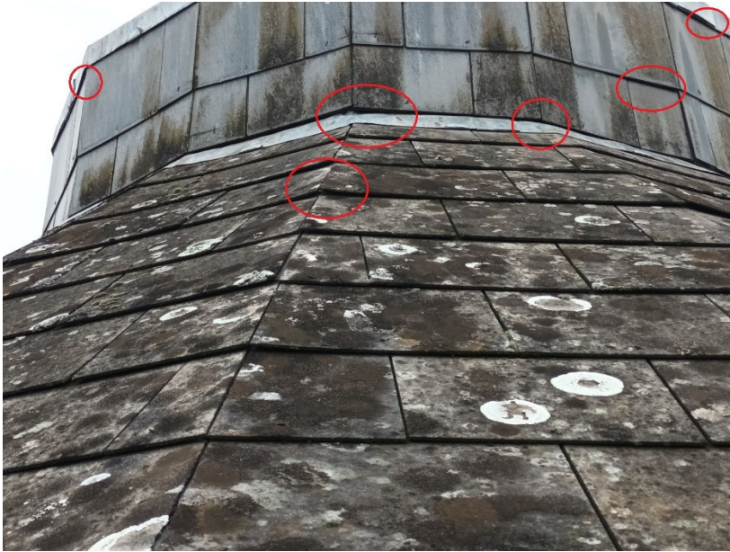
Photo 3. Lifted exterior tiles and lead flashing
