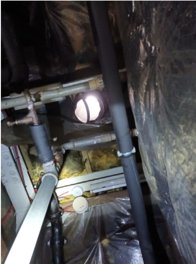
Photo 9. Skylight allowing possible bat entry to the interior
