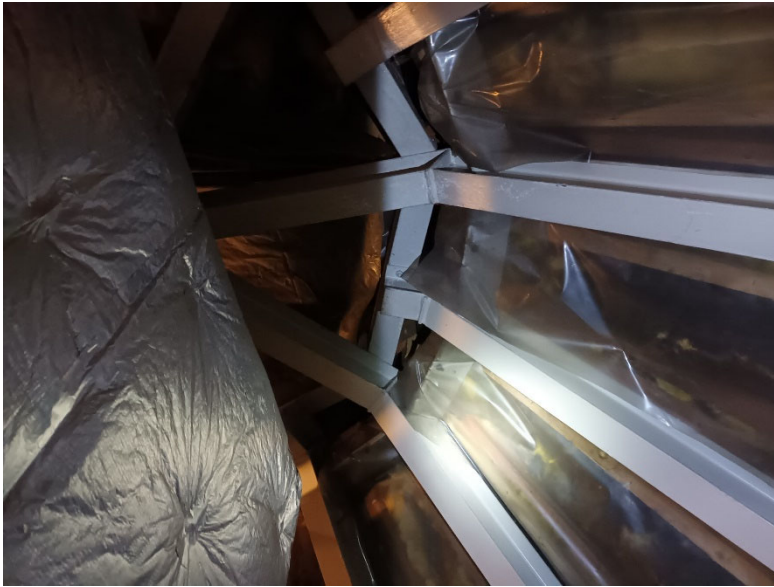
Photo 12. Complexity of interior roof. Abundant crevices and spaces.
