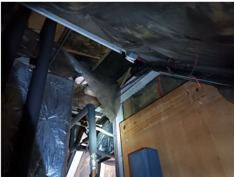
Photo 11. Complexity of interior roof. Abundant crevices and spaces.
