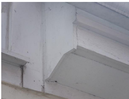
6. Timber soffits tight to the rendered walls along the northwestern side of the bungalow.
