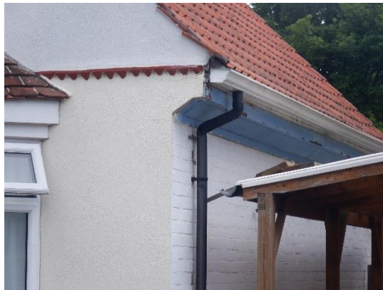
8. A gap present between the paintwork and timber soffit in the rear northern corner.
