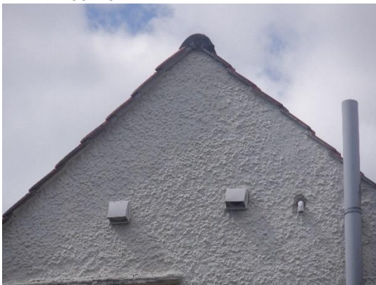
9. Verge tiles tight to the rendered wall to the rear of the property.
