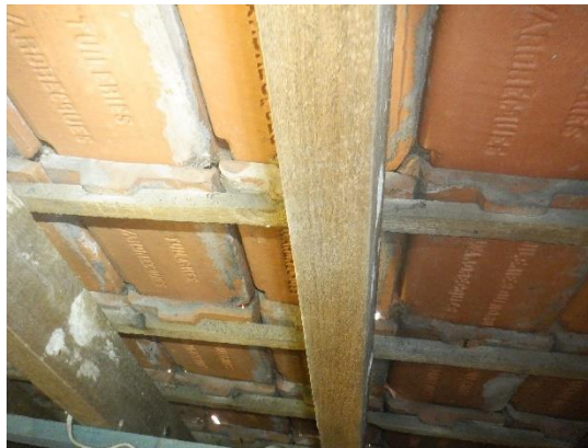
14. The unlined roof with undersides of the roof tiles exposed.
