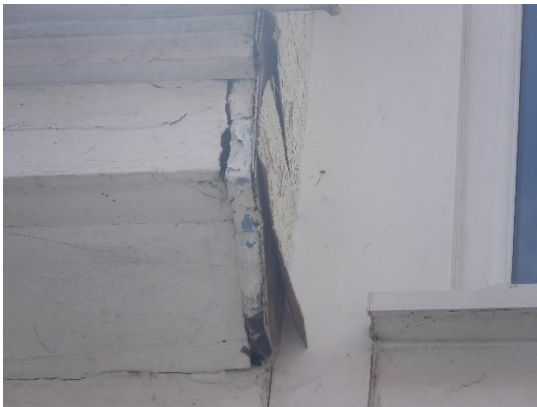
7. Gap in the mortar with further mortar visible behind at the front southern corner.
