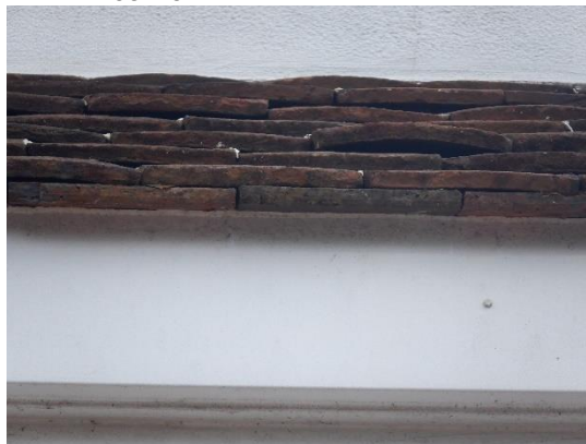
10. Roof tiles uneven on the bay window to the front of the property.
