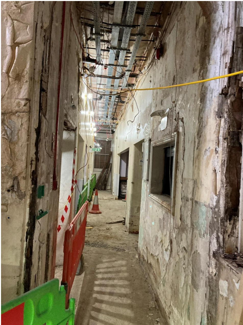
Plaster damage in the ground floor at the north end
