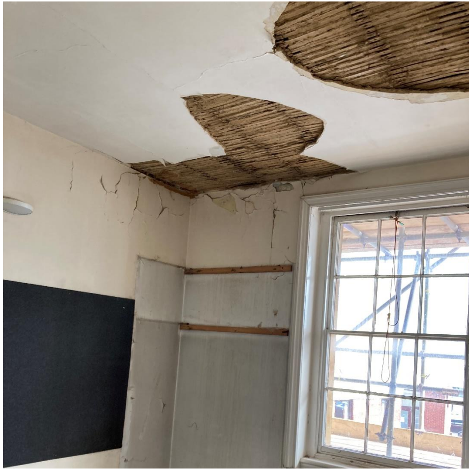
Lath and plaster ceilings are generally damaged
