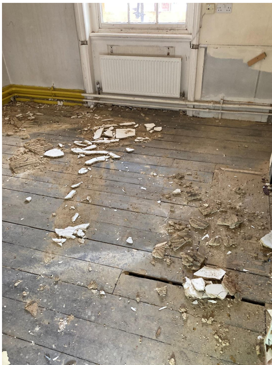
Typical boards on the second floor
