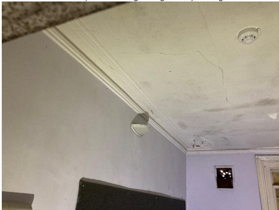
Cornice remains in a few locations on the second floor
